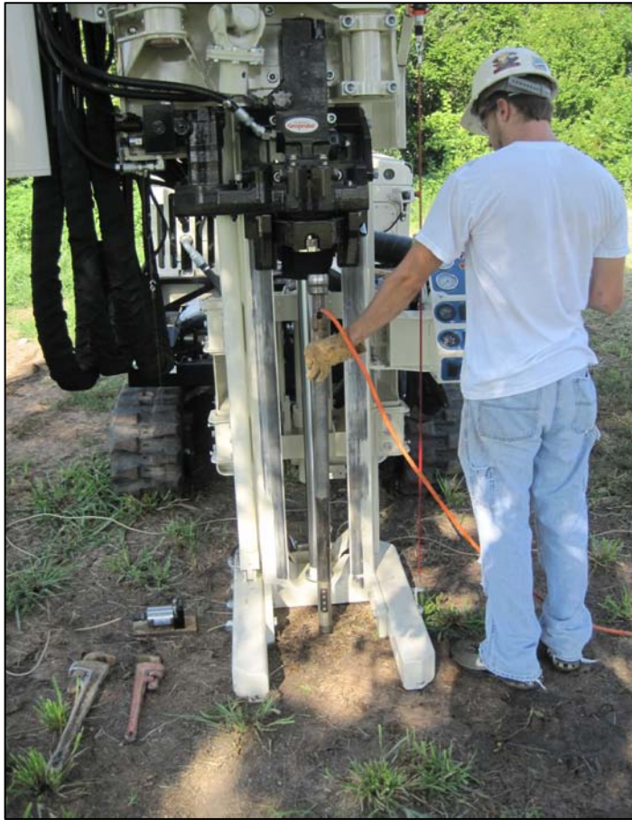
Figure 2: Operator setting up HPT Probe for advancement into the subsurface with a Geoprobe® 7822 machine. The HPT probe is advanced at 2cm/sec using the system hydraulics and probe hammer when required. Logs to a depth of approximately 60ft (20m) are usually completed in about one hour.
