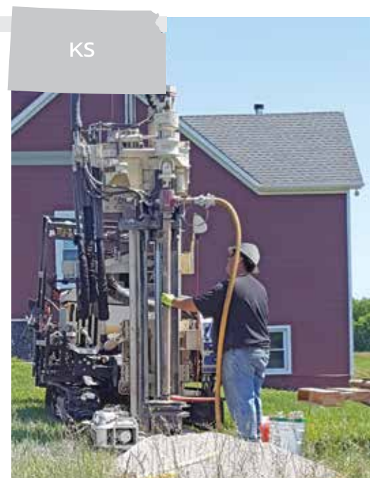
Installing geothermal loops in 6-inch diameter, 150-foot deep bores with a 7822DT using an industry-standard drill rod with a side-port swivel connected to rotary head. An external air compressor was used to clean cuttings out of boreholes and activate downhole hammer.
