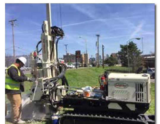
Cory Walker, with CORTEK Drilling in Spring Hill, TN, is installing monitoring wells using air rotary drilling methods.
