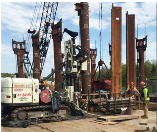
(l to r) Randy Crandell (at the control panel), Chris Ruschmeyer, and Shaun Biggs used an 8140LC rotary sonic to advance 6-in. casing to complete all of the sampling and nested well installation work, completing the job 3-1/2 weeks ahead of schedule.
