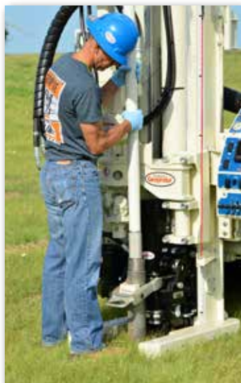
Setting a Geoprobe® 2.0 in. Slim Prepack using 3.75-in. tooling and a 7822DT.
