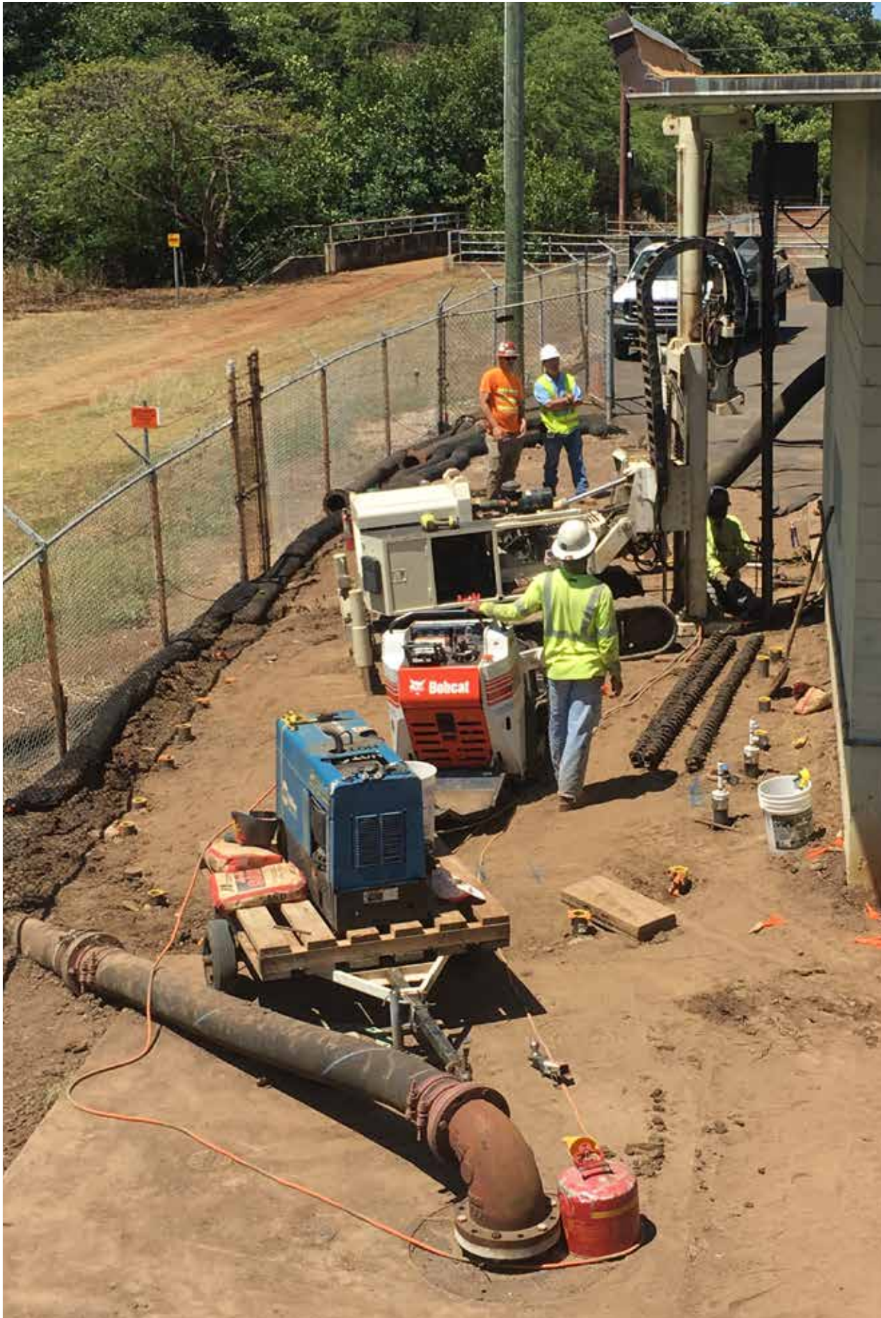
GeoTek was selected for the work because the 6620DT allowed pipe installation under the overhang and without the removal of the fence. Neither criteria could be met by competitors who don't own Geoprobe® equipment. The installation layout can be seen encompassing the equipment.
