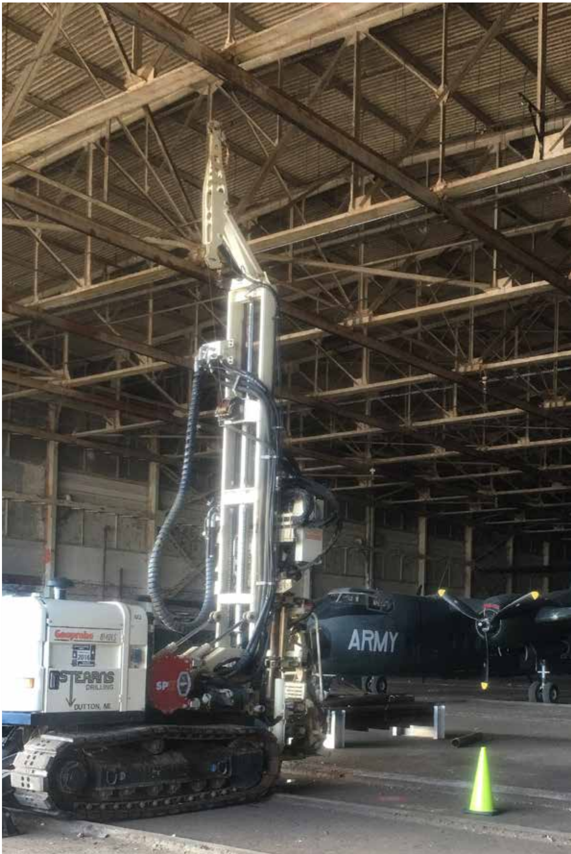
The Stearns Drilling 8140LS Rotary Sonic sets up inside one of the production buildings at the former Willow Run Powertrain Plant in southeastern Michigan for soil sampling and monitoring well installation. In the background sits a DeHaviland DHC-4 Caribou.
