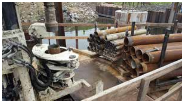
Major Drilling used their 8140LC with 6x8 sonic casing. Continuous soil sampling below the water was completed with a 4-in. core barrel.
