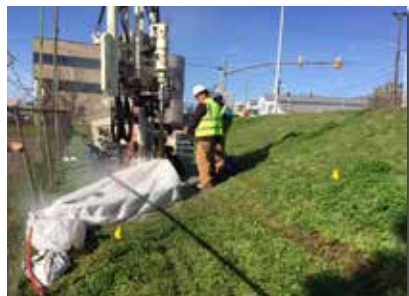
Using a special enclosure to minimize escaping dust, a 7822DT is used to install monitoring wells in a roadway right-of-way. Air rotary drilling was a feature that convinced the machine's owner, Cory Walker, CORTEK Drilling, to purchase the machine.
