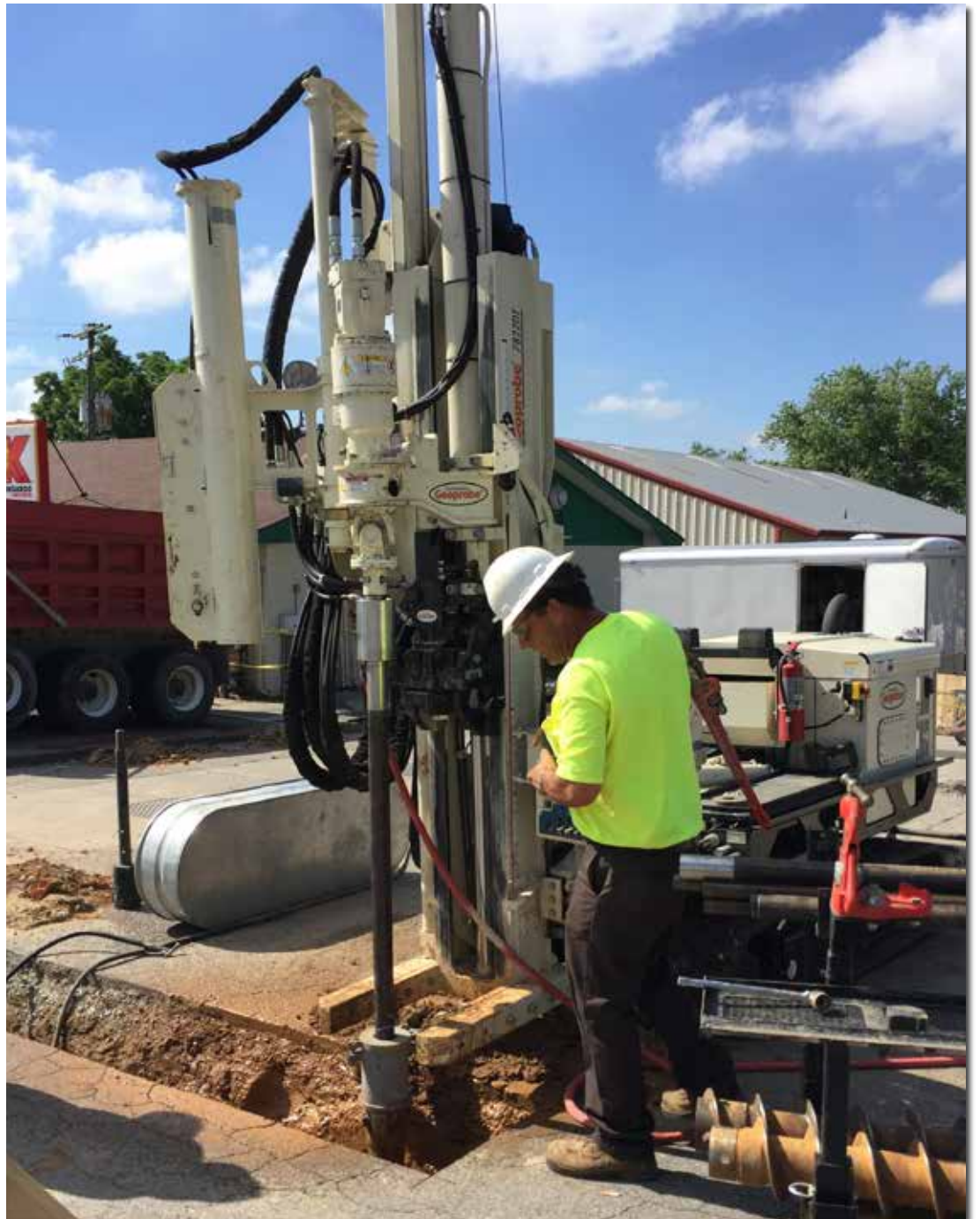
A Geoprobe® 7822DT, connected to an air compressor, is used to install monitoring wells at an underground storage tank site by Cory Walker, Owner of CORTEK Drilling.
