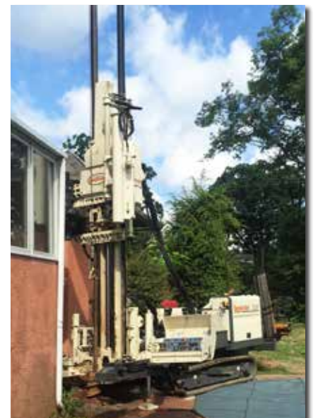
One tight area! Active Environmental experienced just how versatile the 3230DT rig can be by snugging up to a residence to install a monitoring well.
