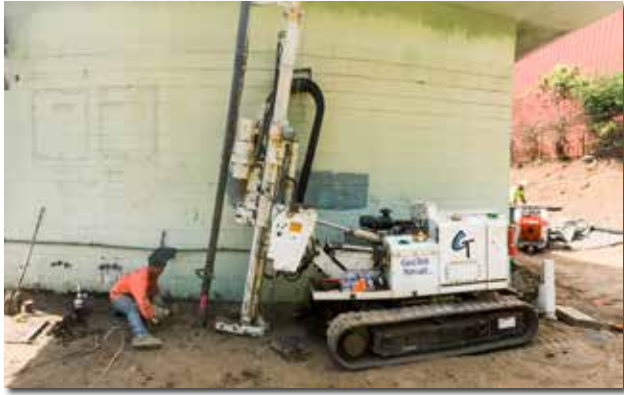
Drayko welds two sections of pipe together under the overhang of a pump station. The maneuverability of the 6620DT permitted a battered installation under the buried sewer main to ensure a 'solid' frozen curtain.
