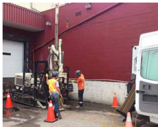
CJ, Driller, and Dallas, Helper, running LL-MIP with Matrix Environmental and JFM Environmental Ltd.
