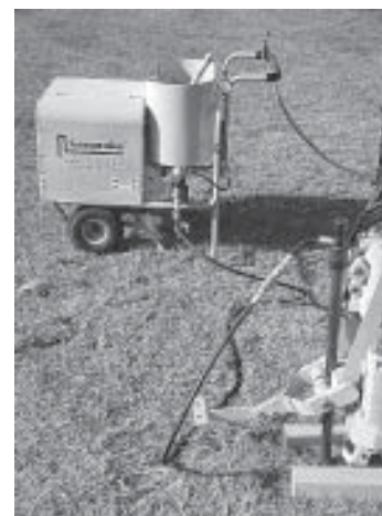
The GS1000 Grout machine connected to the tool string with the high-pressure hose (GS1052) and grout pull cap (GS1254). Using the rod grip puller (GH2150K) makes the retraction grouting easy and quick.
