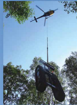
The track section of the 6712DT is lowered to a site on the mountainside to advance 4.25 in. hollow stem augers to install 2.0 in. monitoring wells.
