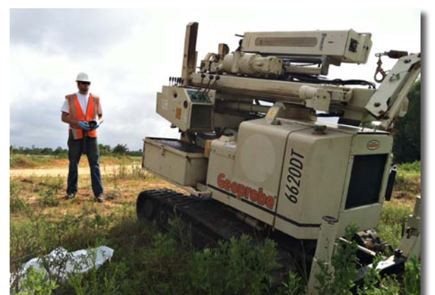
The remote control is utilized to maneuver the rig into difficult terrain.
