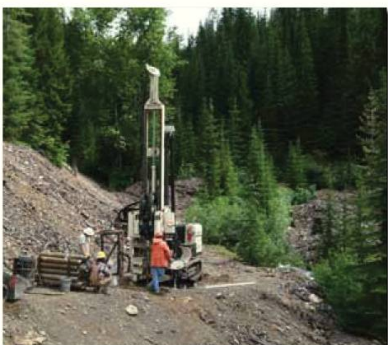
Major Drilling Environmental uses and 8140 Rotary Sonic for remote sonic drilling within mine rock dump in northern Idaho. (see related story on pg. 8.)
