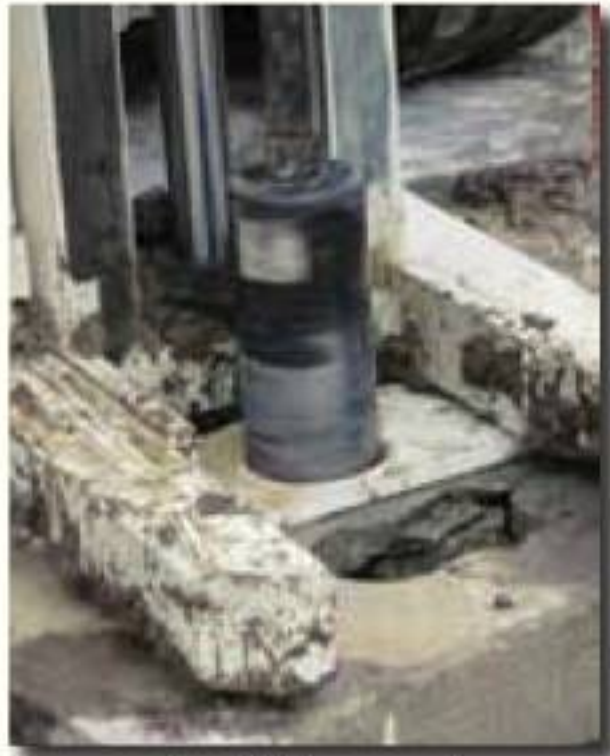
Concrete coring with the two-speed, bi-directional rotation feature of the GH64 Hammer on a 7822DT.
