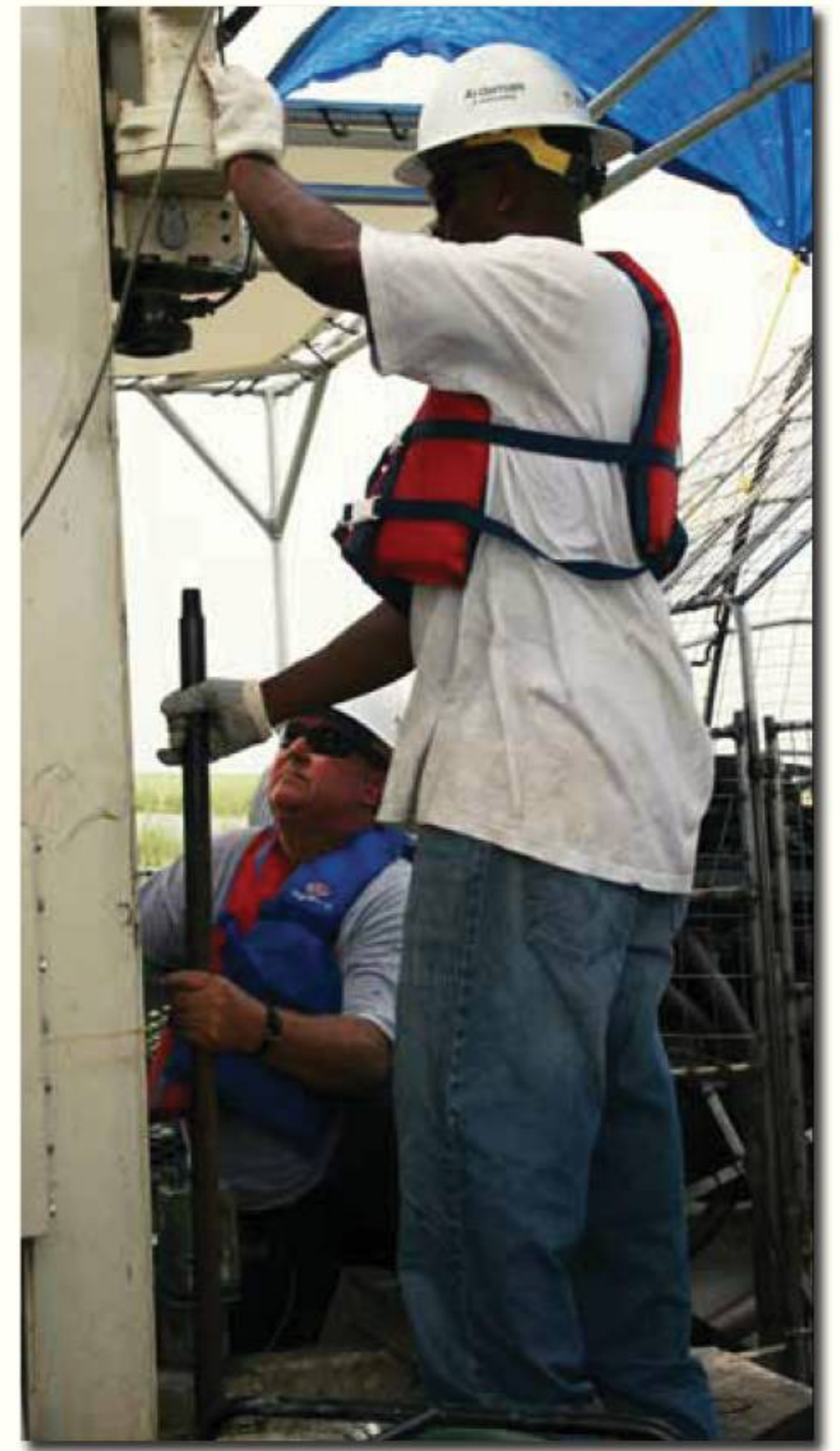
Jermaine George, Ardaman Associates Driller, and Dempsey Thibodaux, Senior Driller (kneeling), push a CPT cone to 200 ft. during the 6-month-long Port Fourchon project in Louisiana marshland.
