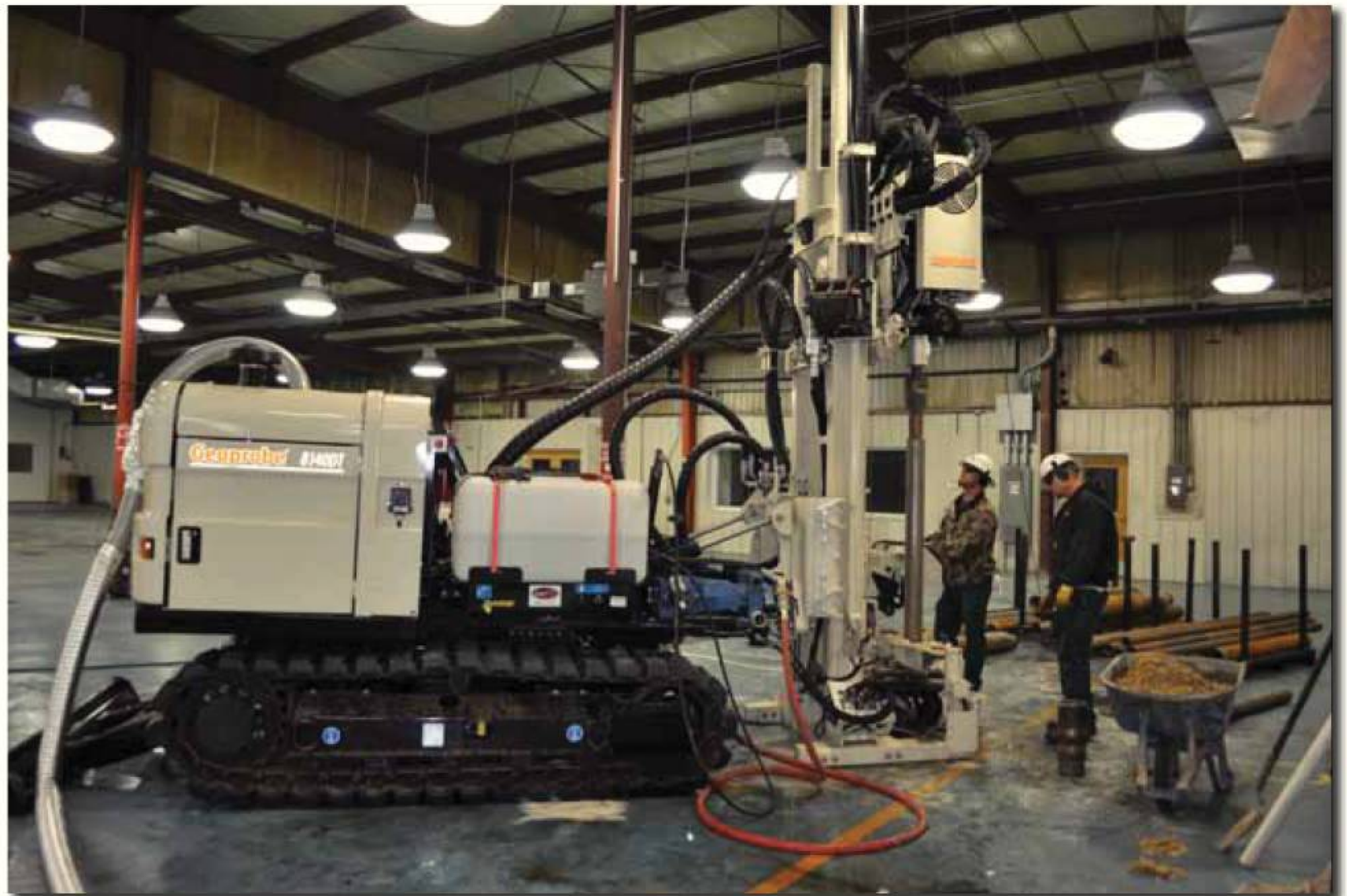
The Huss Drilling field team from Dade City, FL, uses the 8140 Rotary Sonic to install a monitoring well to nearly 100 ft. (see related story on pg. 9.)
