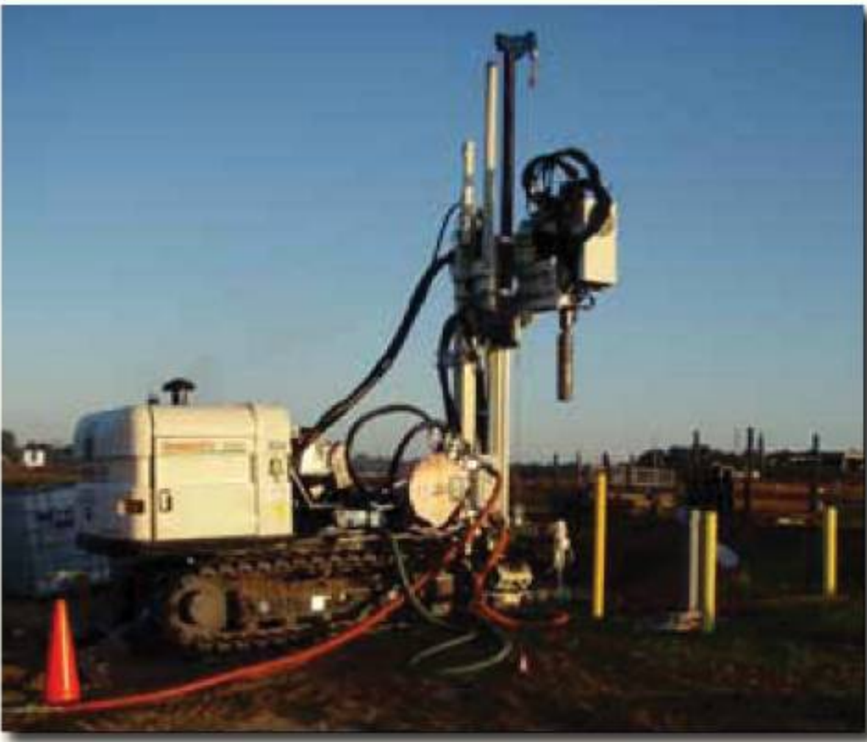
(above) MDE uses an 8140 Rotary Sonic for drilling and installing 4-in. stainless steel wells in north Florida. Sixteen wells were installed to depths ranging from 45 ft. to 90 ft. deep each.
