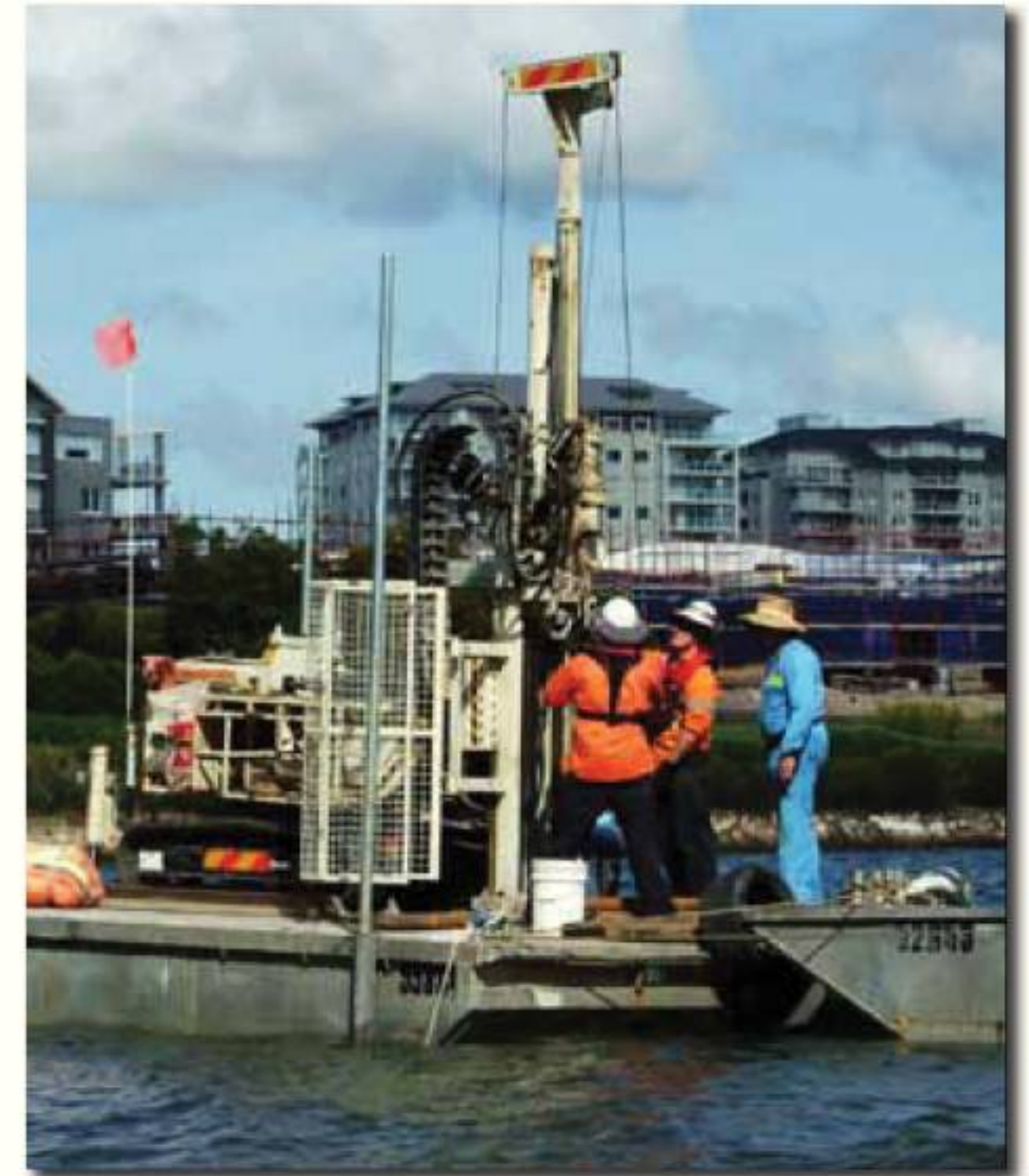
The Terratest team relied on the DT325 tooling to continuously sample all locations in the harbour to bedrock. This tooling resulted in very little disturbance of the sediment during sampling.
