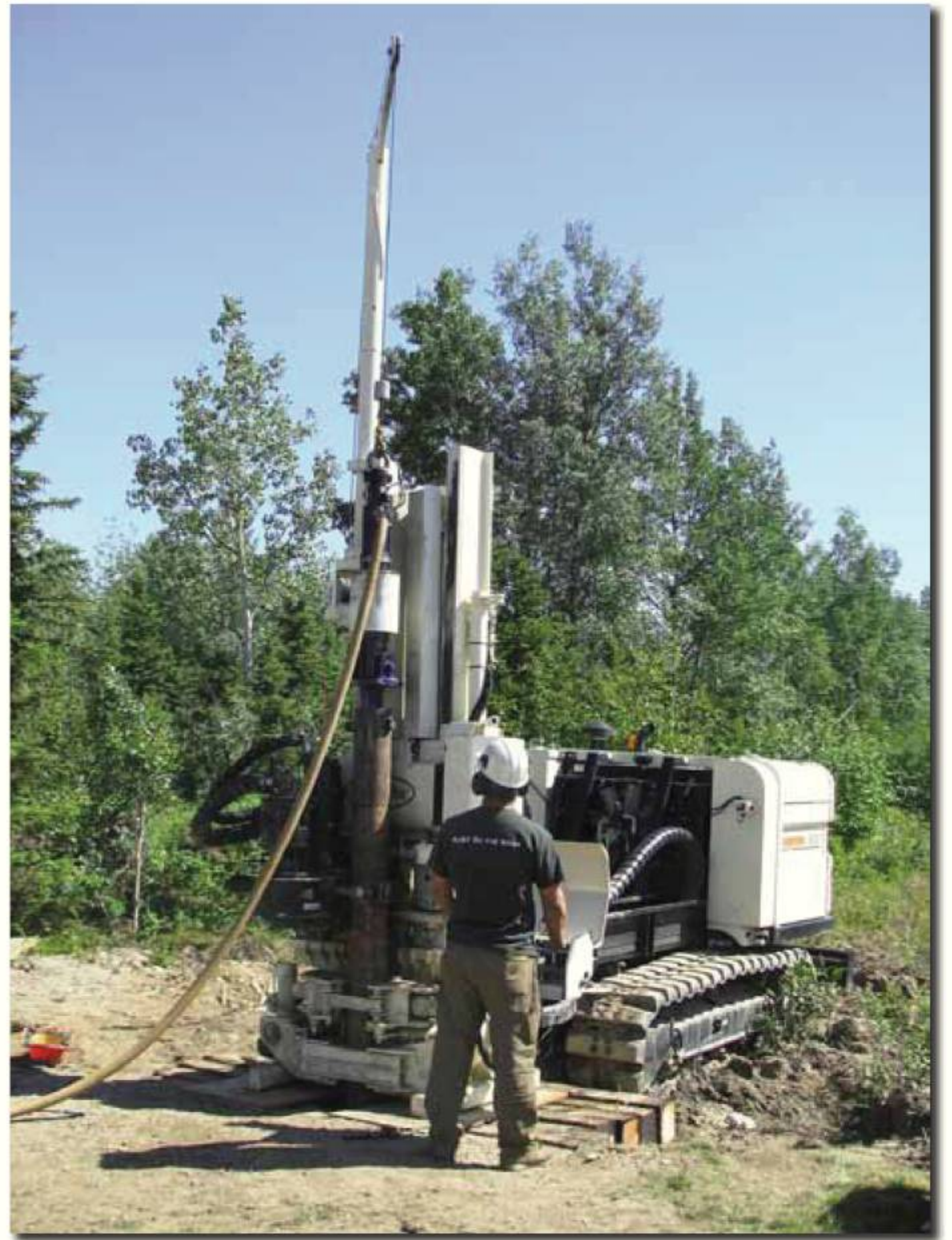
An 8040DT, owned by GeoTek Alaska in Anchorage, AK, works at an old coal mine.
