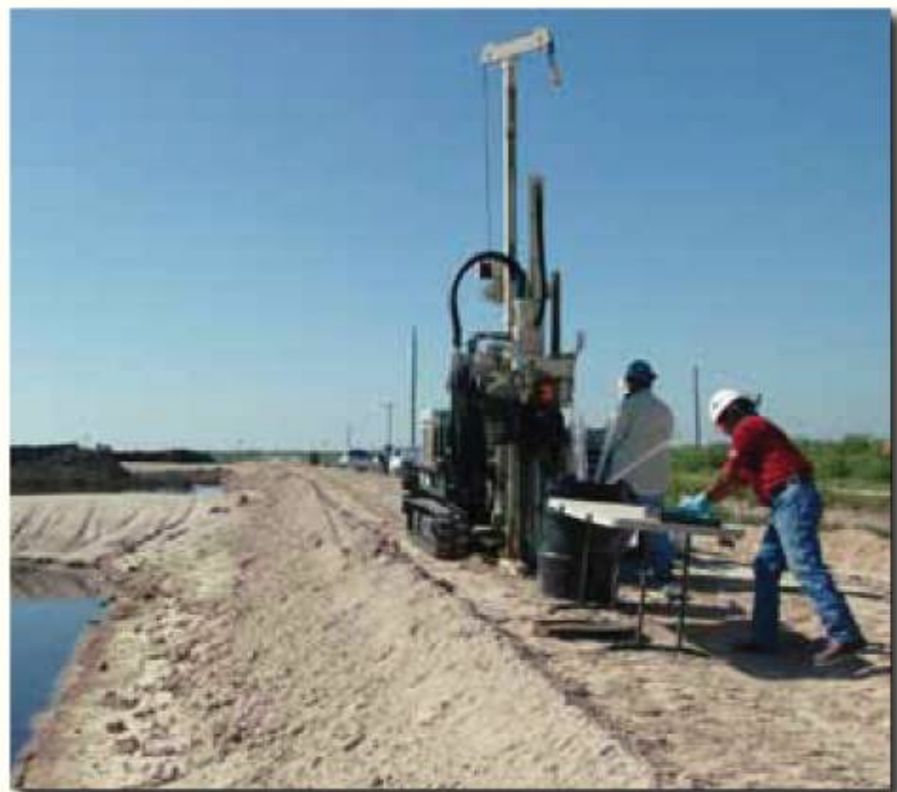
Vortex Drilling in San Antonio, TX, use a 7822DT to install temporary monitoring wells along the perimeter of a wastewater lagoon.
