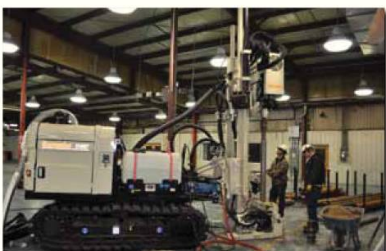
The Huss Drilling field team for the project, Kent Fowler, Driller and Tony Hudson, Operations Manager, use the 8140DT Rotary Sonic to install a monitoring well to nearly 100 ft. In spite of completing most of the work inside warehouse buildings, the mid-sized sonic rig was able to easily work inside the low overhead clearance facility.
