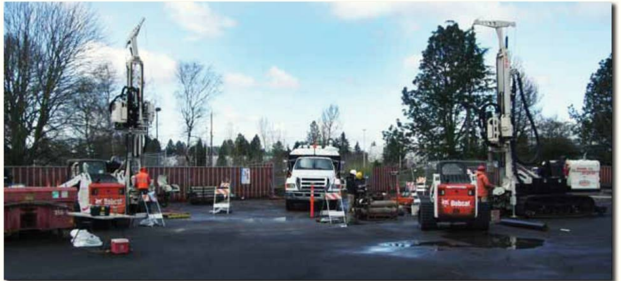
Two of MDE's 8140LS rigs installing remediation electrodes in Beaverton, OR, using 10.75 in. OD casing.
