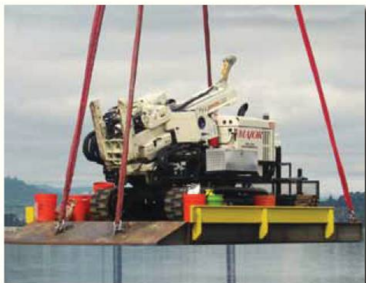
Major Drilling Environmental in Portland, OR, along the Willamette River in Oregon lowering their 7822DT to the worksite.
