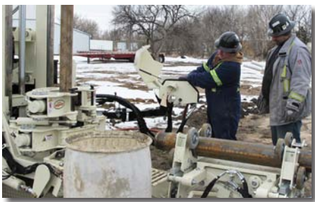
Clayton Duralia (left) and Bobby Tura, with Omega Environmental Drilling, control the movements of the rod handling equipment on the 8140LS.
