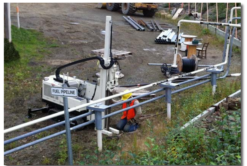
DJ Wardwell uses the 54LT to collect MCS soil samples near an active above-ground fuel line at a site at Indian Mountain in Alaska.
