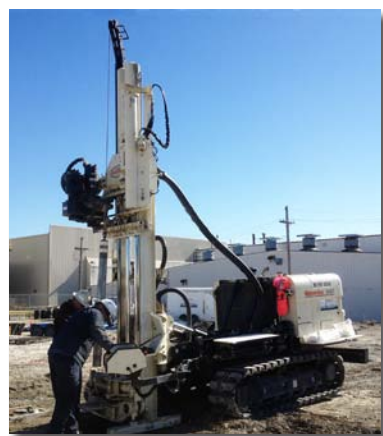
Drillers Pat Seymour and Brian Schilling use the 8040DT at Lambert International Airport, St. Louis, MO, to install 2-in. double cased wells utilizing Geoprobe® DT45 casing.
