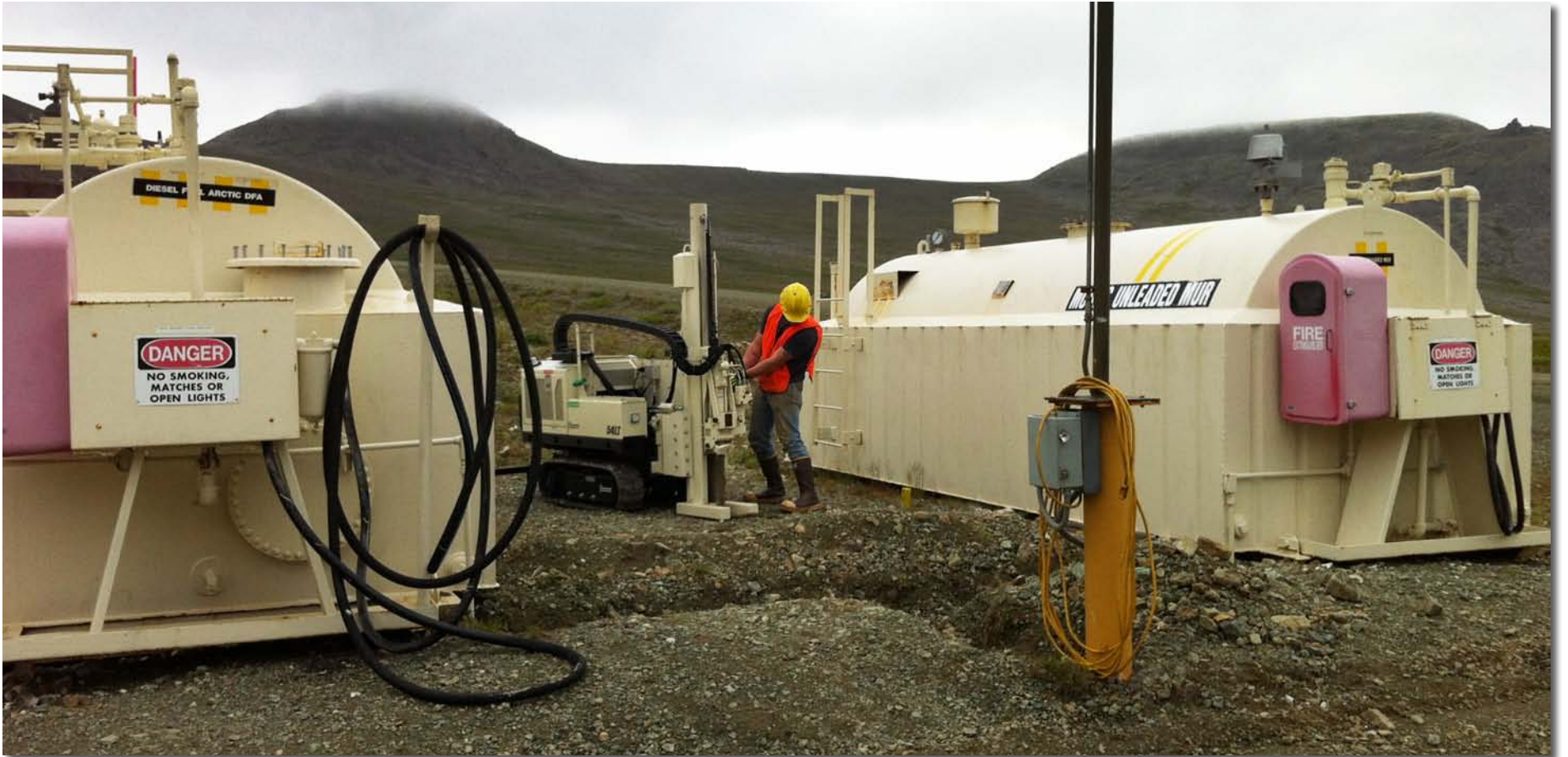
Collecting MCS soil samples between two active fuel storage tanks at Cape Newenham Air Force Station Long Range Radar Site (LRRS) in southwest Alaska.
