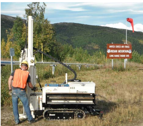
DJ Wardwell with Discovery Drilling uses the 54LT to collect soil samples at Indian Mountain Air Force Station in Alaska near the top of the runway.
