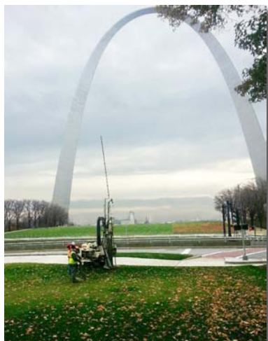
Driller Shawn Seymour and Helper Joe Luberda run the 6610DT in St. Louis, MO, in the shadow of the Gateway Arch. This rig and the REDI 6620DT are used a lot for sampling and augering for installing monitoring wells.
