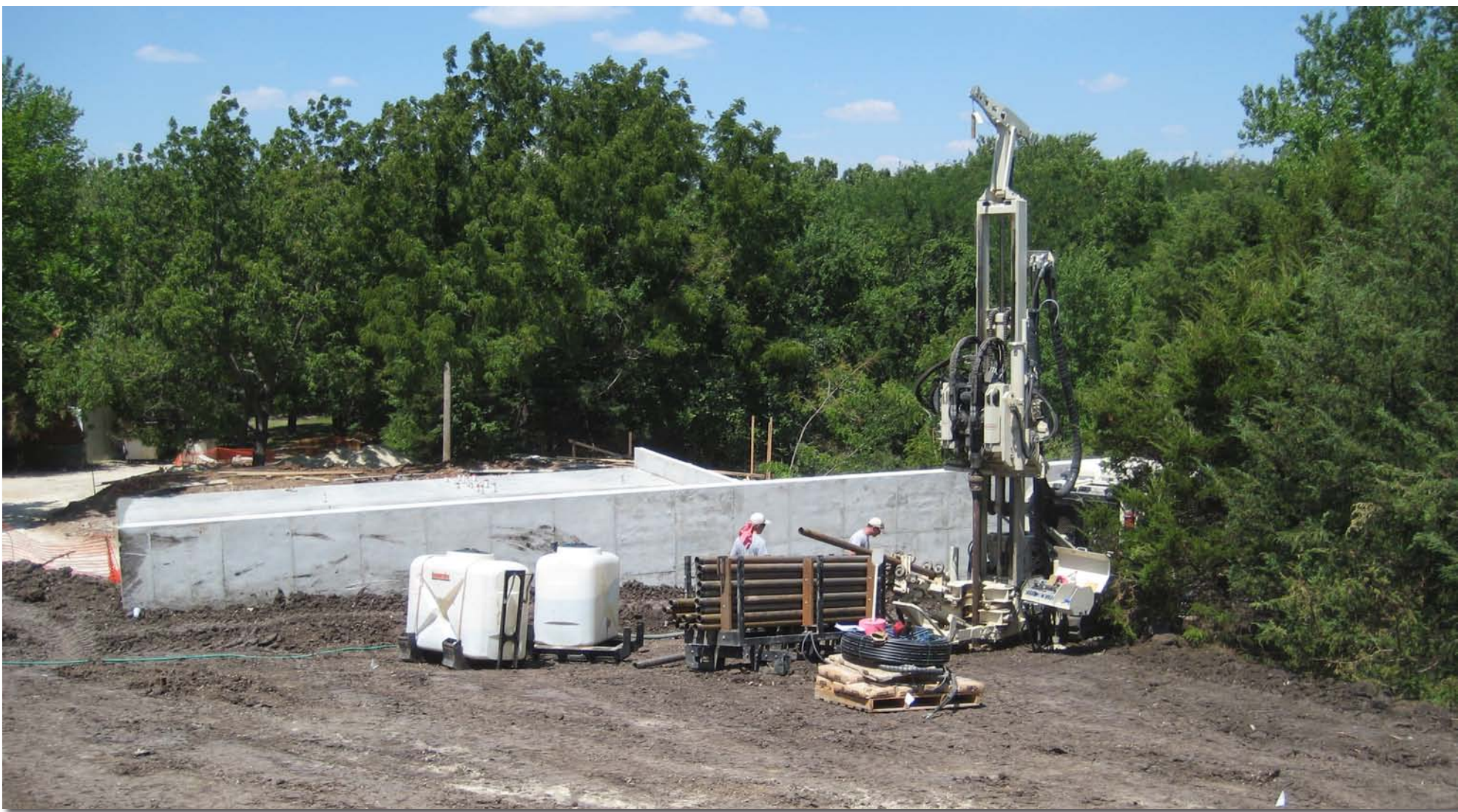
A Geoprobe® 8140LS Rotary Sonic works at a geothermal loop installation site near Florence, KS.
