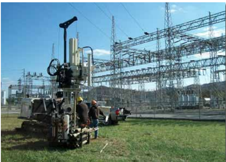
The EnviroProbe field team use their 8040DT with DT45 and MCS tooling to install four temporary piezometers at a site in West Virginia. Operating the rig were Dale Kestner (left), Driller, and Chris Henderson, Field Services Manager.
