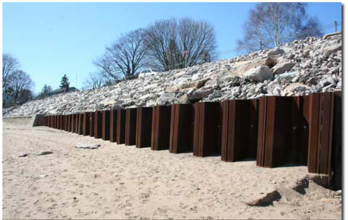
(above and below) The sea wall at Branford, CT, is shown after repairs were made when Hurricane Irene destroyed the sea wall last August.
