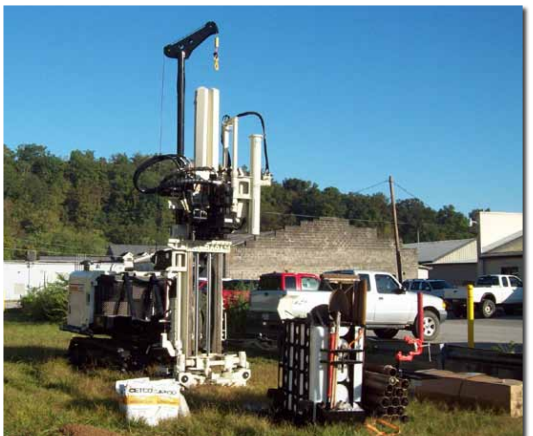
Two-inch monitoring wells are being installed at this residential area using DT45 tooling and the 8040DT.
