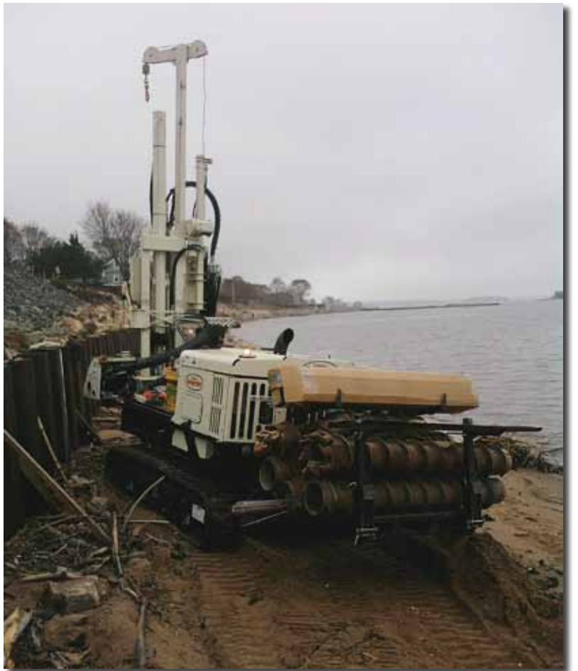
The 7822DT, with Floyd Cross, Driller for American Environmental, at the controls, took DT22 samples along the destroyed sea wall in Branford, CT. The task was to identify the depth to competent rock so repairs to the wall could be designed and constructed in a short amount of time. Because of its compact size and light weight, the 7822DT was able to drive along the beach without laying tracking pads unlike conventional drill rigs.
