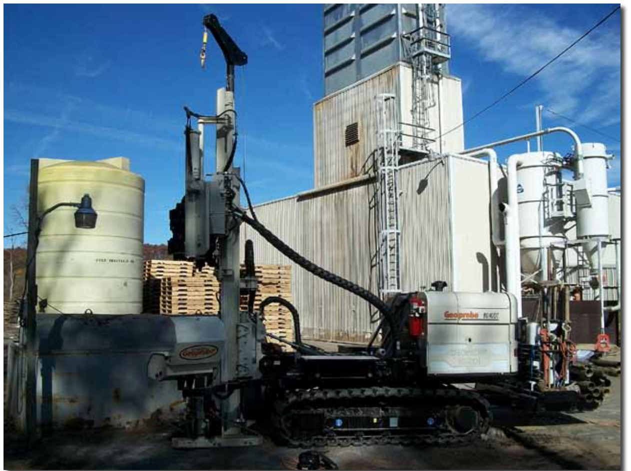
The EnviroProbe 8040DT pairs up with DT45 tooling to collect soil samples at an abandoned grain handling and storage facility in West Virginia.
