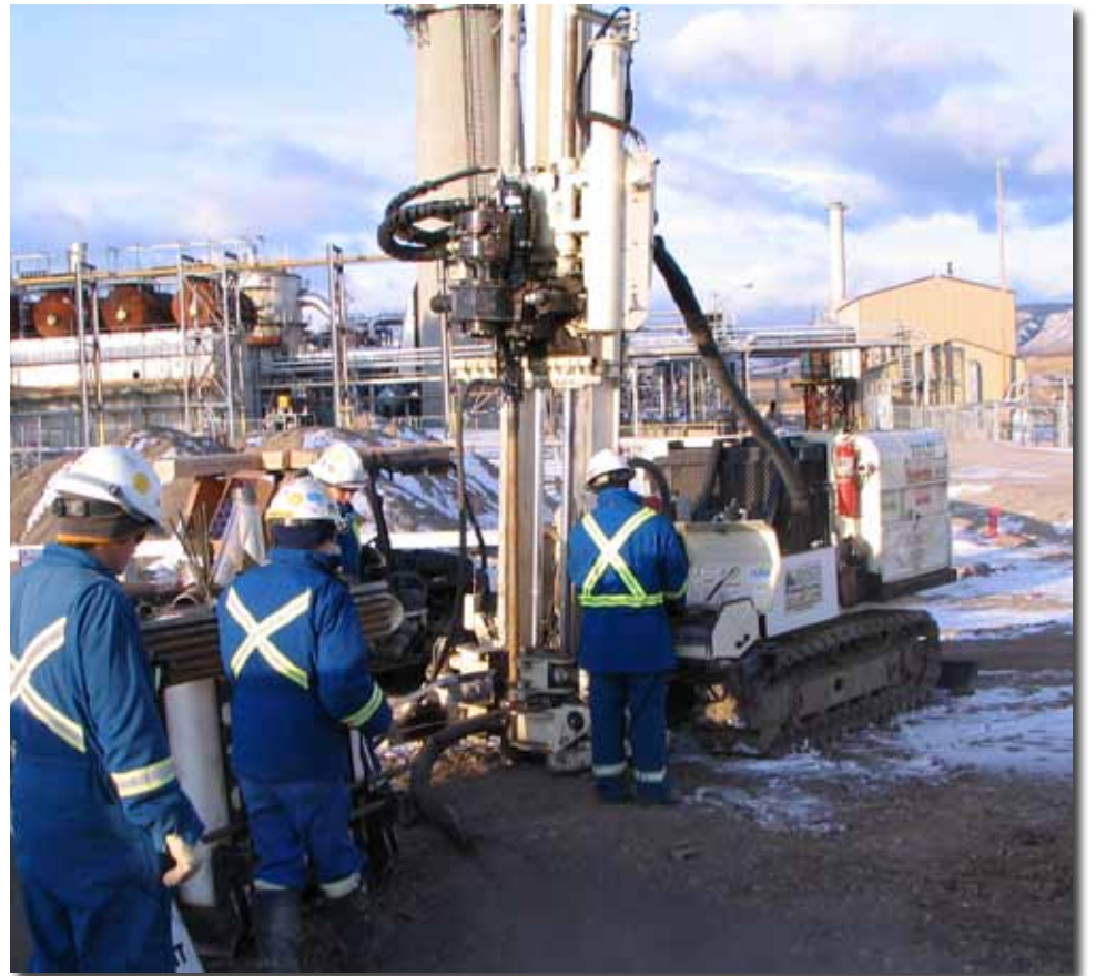
Air rotary drilling was used with the 8040DT to advance casing for monitoring well installation at a site in southwestern Alberta in Canada. Assisting Jordan Ernst (right), Driller for Ernco, was Brett Nixey (left of rig), Driller's Assistant. Two representatives of the consulting firm appear to the left.
