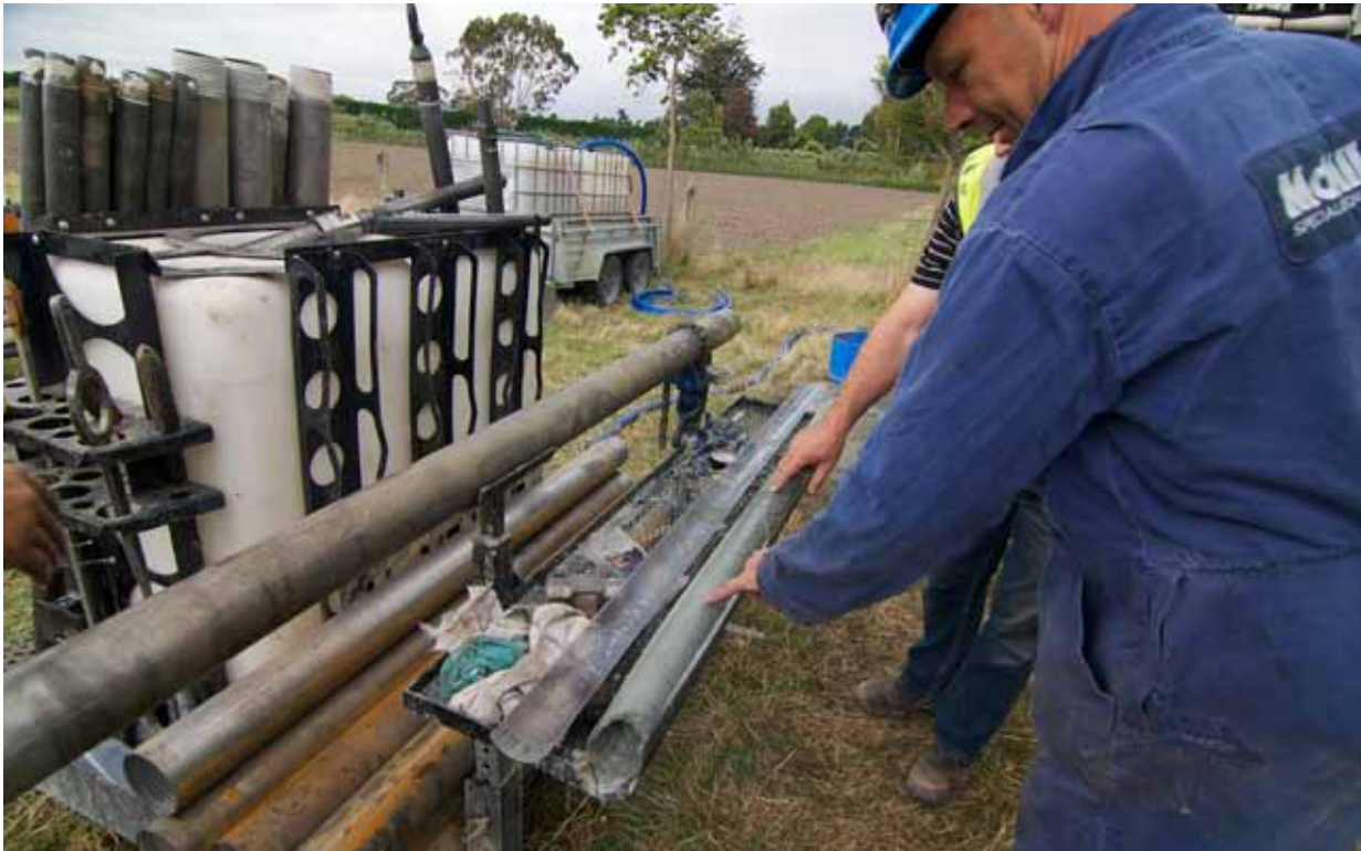
(above) The McMillan Drilling field team maintained 100 percent sample recovery throughout their project using the DT45 system and their 8140LS rotary sonic, drilling to depths of 75 ft. SPT test were conducted at 5 ft. intervals.
