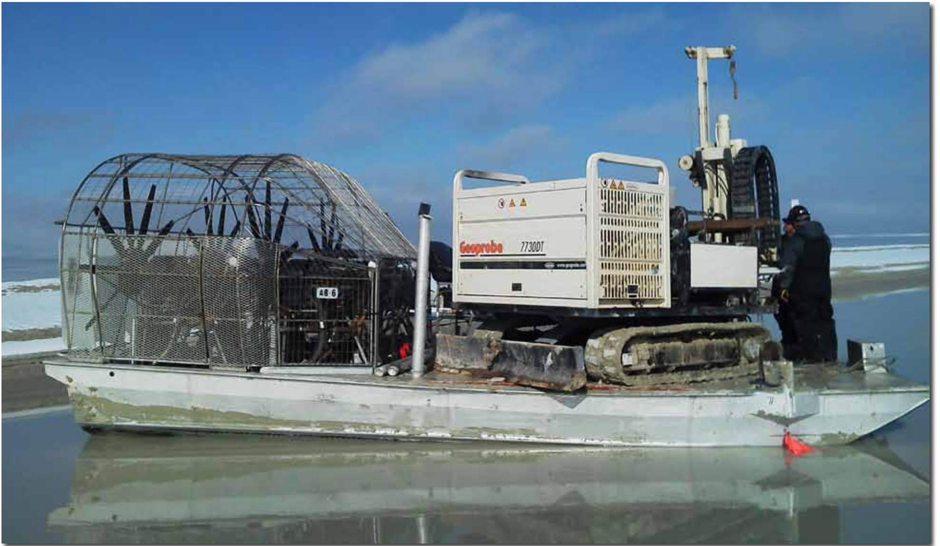
Selected for its compact size and dependable power, Darin Bromley (left) and Ryan Roodbol, with Direct Push Services in Salt Lake City, use the Geoprobe® 7730DT to collect soil cores and install temporary piezometers at over 400 locations for a mineral exploration company.
