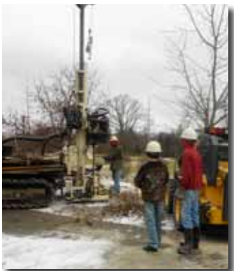
(above) Stevie Govan (brown jacket) works with his brother, Will, while their dad, Dean Govan uses an 8040DT to install a backup well at the family home.
