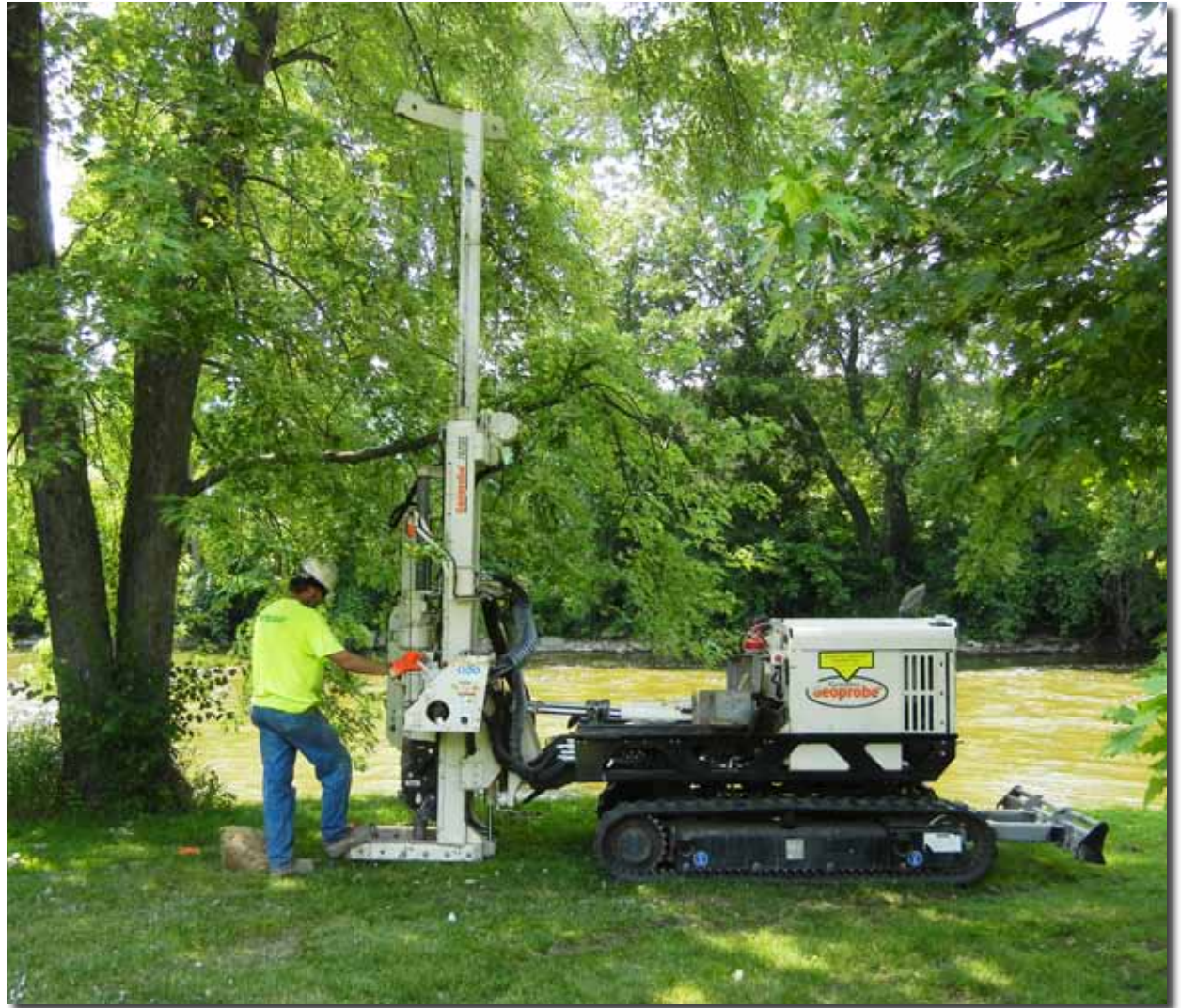
Dave Breede, Drill Operator for Raimonde Drilling, works at a location where a light-weight and portable drill rig was requested by the client. The project was completed without disturbing the riverside park’s natural grasses and mature foliage.
