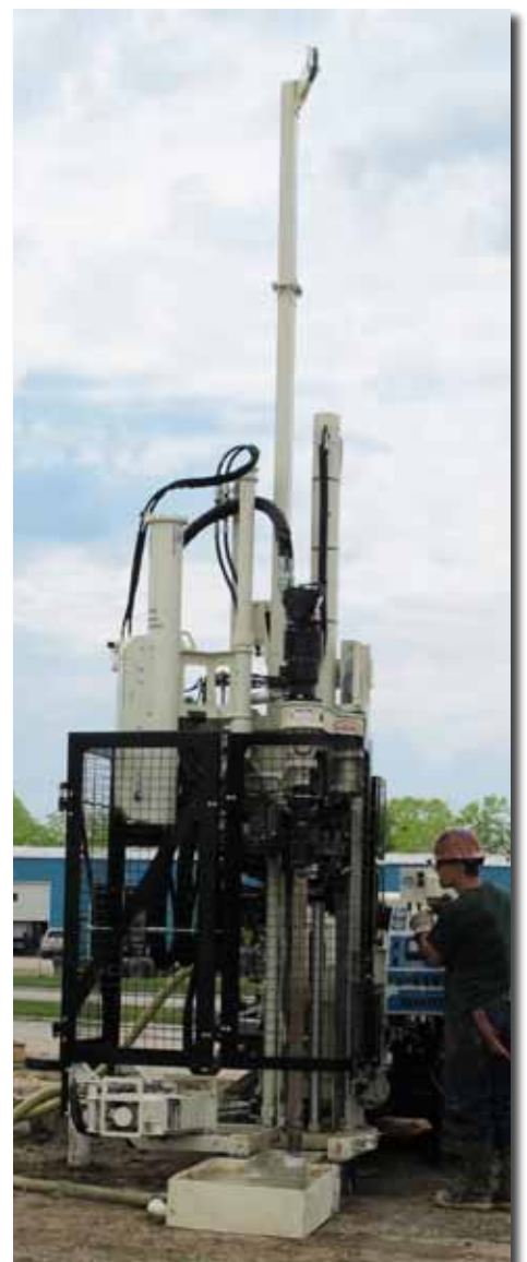
Quinton Wilson uses the 7822DT equipped with a new interlocking Rotational Safety Cage with a GA4000 Auger Head. He was setting 4.5 in. conductor casing in preparation for wireline coring.
