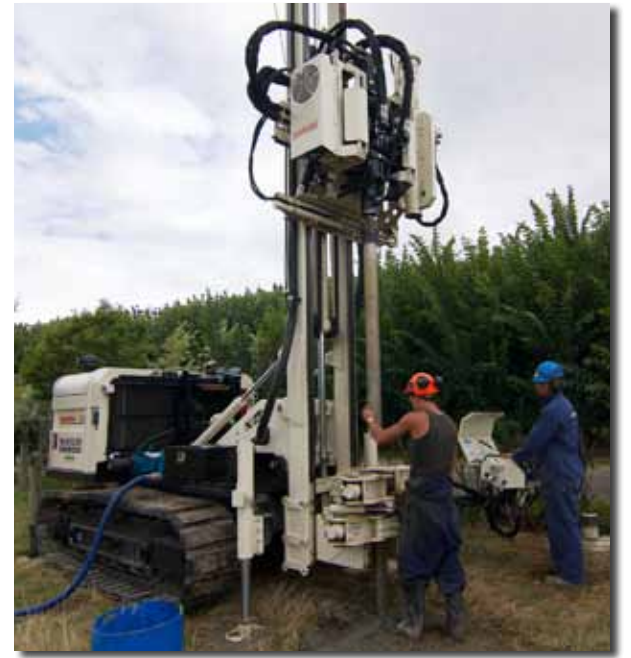
McMillan Drilling Services is on site with their 8140LS (long stroke) rotary sonic rig in Canterbury, New Zealand. The field team used the DT45 sonic sampling system for the geotechnical work.
