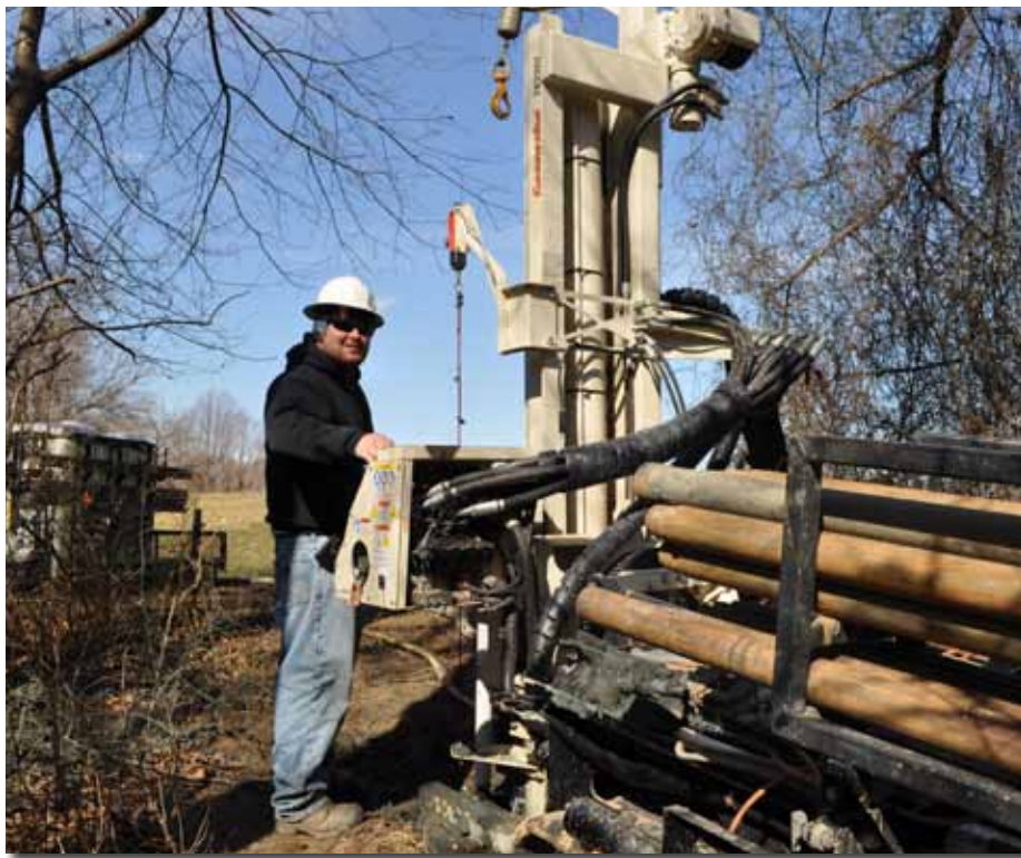
A.J. Benjamin, Rig Operator for Environmental Probing Investigations, installs 70 ft. deep 2 in. monitoring wells using the 7822DT.
