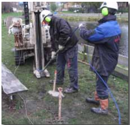
Teamwork by the NIRAS field crew was an essential factor in successfully completing the MiHpt demonstration in Skuldelev under budget. Here, Peter Thompsen (left) and Thomas Layborn prepare to install the next probe rod to continue advancing the MiHpt probe to depth.
