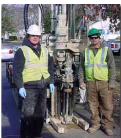
Todd Morgan (left) and Zach Callahan use the new MiHpt logging tool at a residential site in New Jersey.
