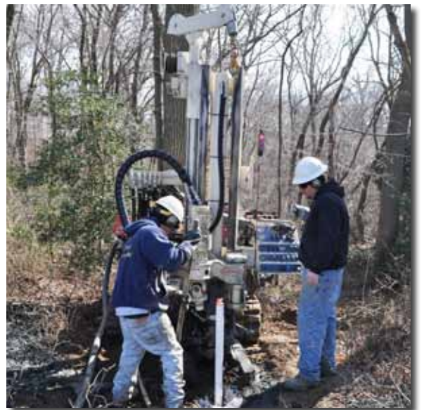
Mike Santore (left) and A.J. Benjamin install monitoring wells for SHAW Environmental in Burlington County, NJ. The cabled E-stop, next to the control panel, can be accessed by either worker.
