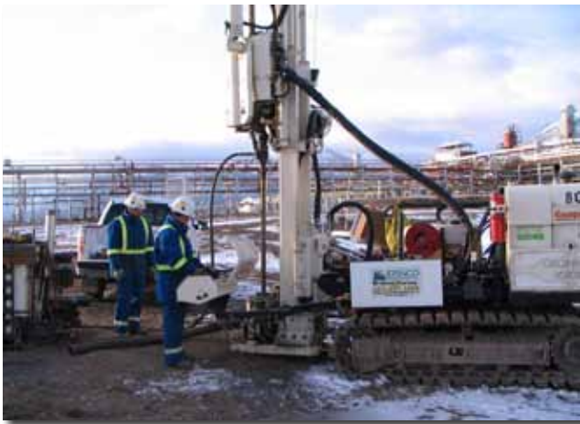
(l to r) Brett Nixey, Driller's Assistant, and Jordan Ernst, Driller for Ernco, use the 8040DT to complete boreholes to approximately 80 ft. for the installation of prepacked screen monitoring wells.
