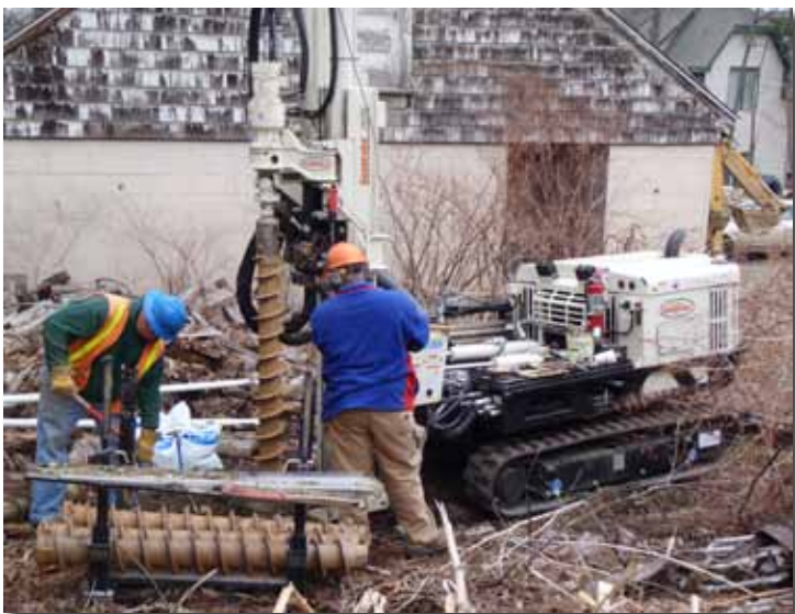
An American Environmental field team uses the 7822DT to set monitoring wells at a site in Connecticut.
