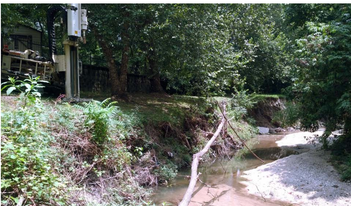
This portion of the Penn Branch Creek shows the deterioration of the gravity walls along the channel. The Penn Branch is located east of Columbia and runs through numerous residential and commercial properties.
