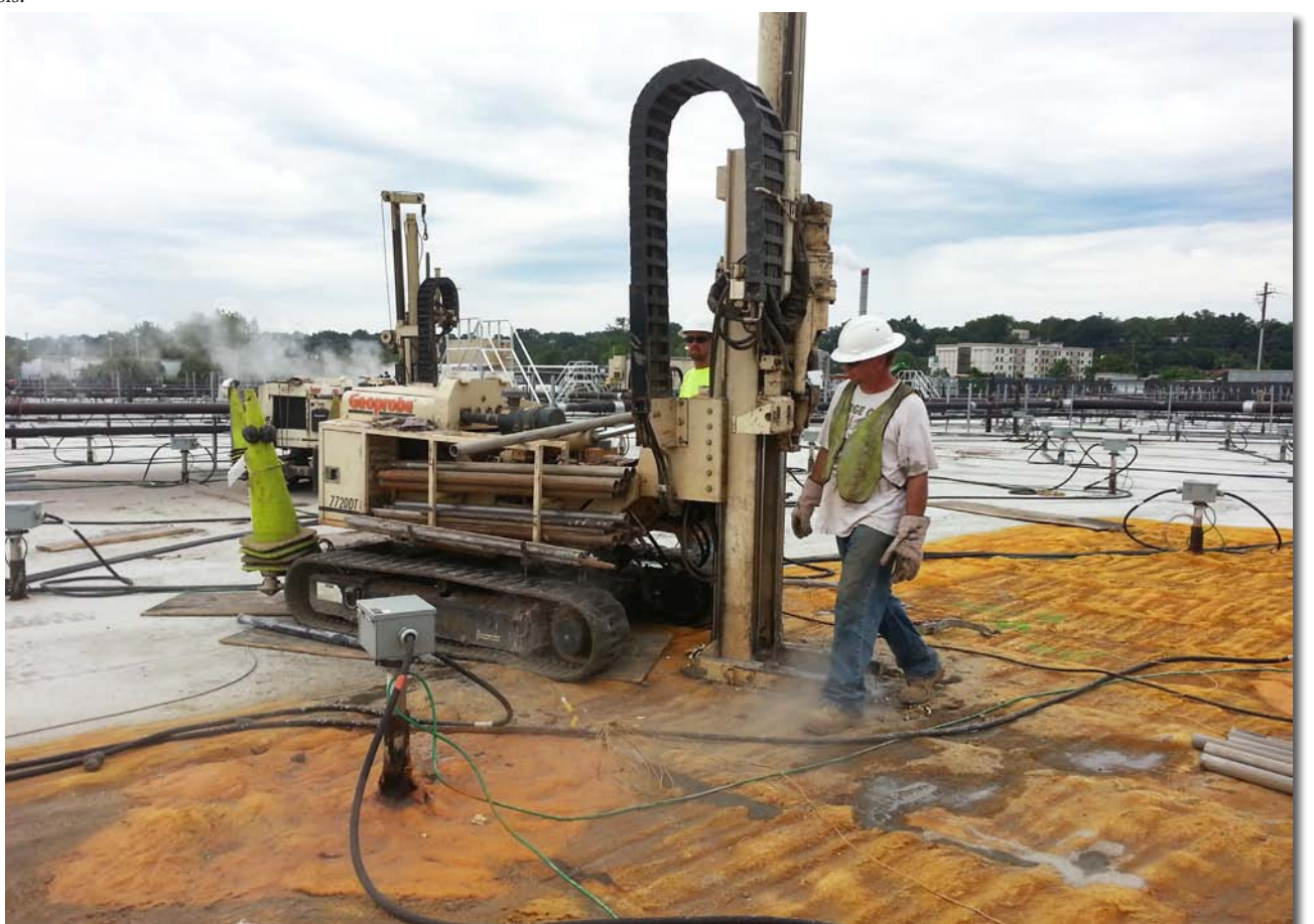
Bob Fleming, EPI driller, with heat-resistant gloves, prepares to collect another soil core. The yellowish-tan material he's walking on is a fine-grained sand that was carried out of the bore holes by the steam.
