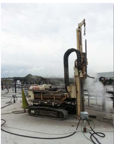
One of EPI's 7720DT rigs stands alone as steam vents from a borehole after sampling while the drillers take a break to get some relief from the heat.
