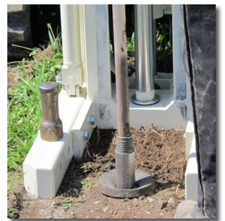
Geoprobe® 2.25-in. probe rods provide the primary driven casing for three soil sampling systems, including the DT22 dual tube system shown here.
