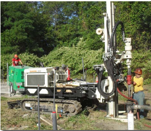
Stone Environmental, Montpelier, VT, uses an air rotary hammer with a 7822DT to install 160 multipurpose injection/monitoring wells at a former drum burial site in New England. The wells were used to delineate the source area of contamination in preparation for an in-situ chemical oxidation remedy.
