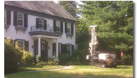
Tri-State Drilling Technologies, in Levittown, NY, uses a 7822DT for residential environmental work.
