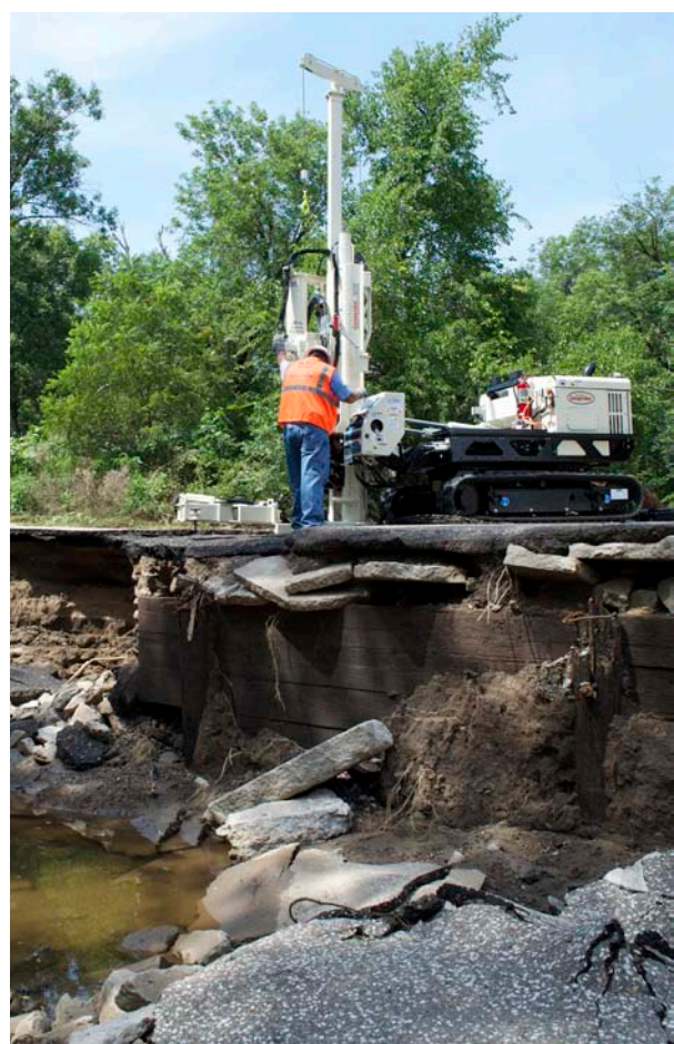
Coring through a variety of underground materials at a disaster site. The power of the compact GA4100 Augerhead performs well for drilling jobs varying from torquing-in hollow stem augers to high-speed rock coring applications.
