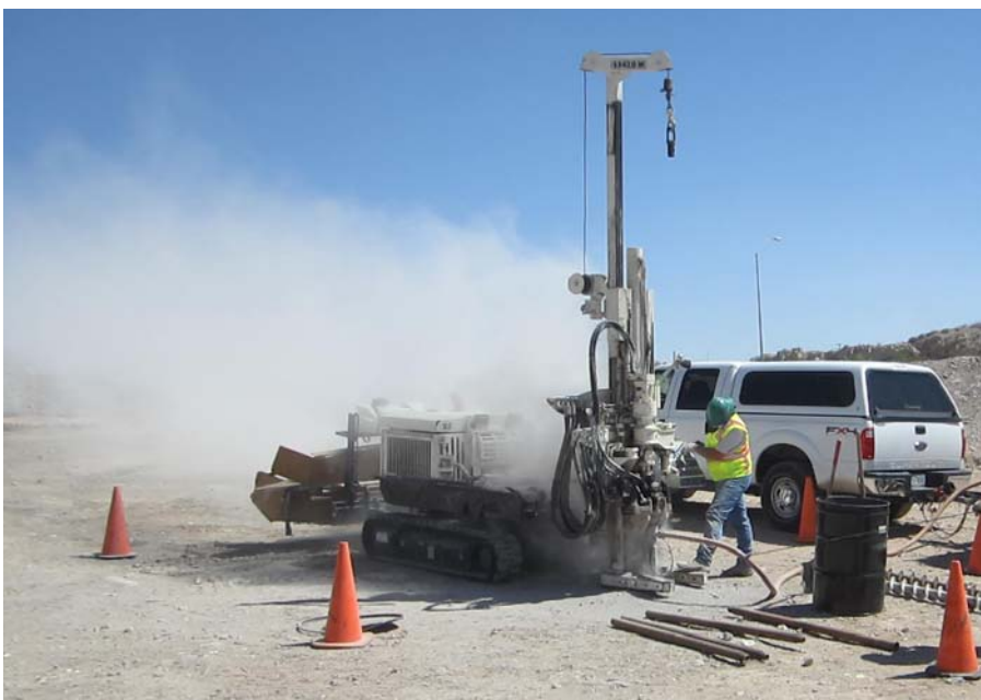
Cody Clayton, with Vortex Drilling in San Antonio, TX, uses an air hammer with their 7822DT on a project in Texas.
