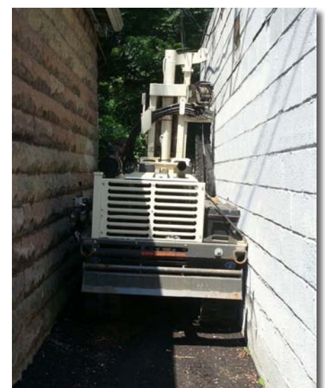
With barely 0.5 in. to spare on each side, the new 6712DT owned by Environmental Priority Investigations in Cream Ridge, NJ, heads "where no rig has gone before!"
