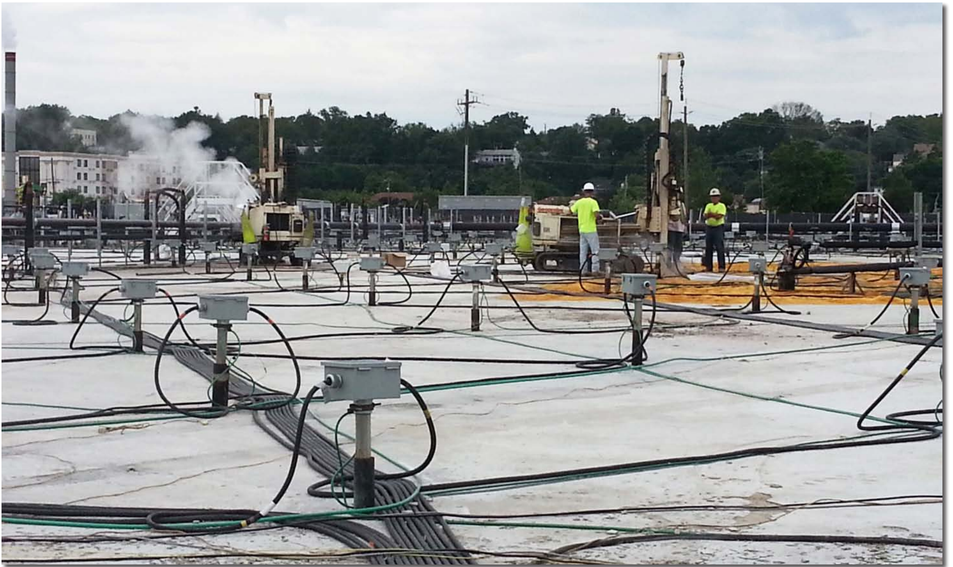
Environmental Probing Investigations collected continuous soil cores from 56 borings at a site in northern New Jersey. The subsurface was pre-heated to nearly 400 degrees F prior to sampling to alleviate onsite contamination. The maze of gray electrical junction boxes and electrical cables and air hoses were used to distribute electricity to power the 'heater cans' in the subsurface.
