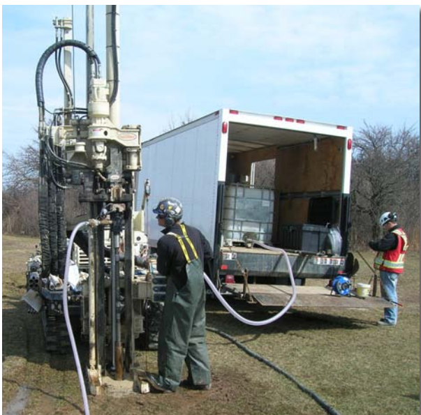
Eric Langdon, Driller/Operator for Strata Drilling, completes another coring hole with the 7822DT.
