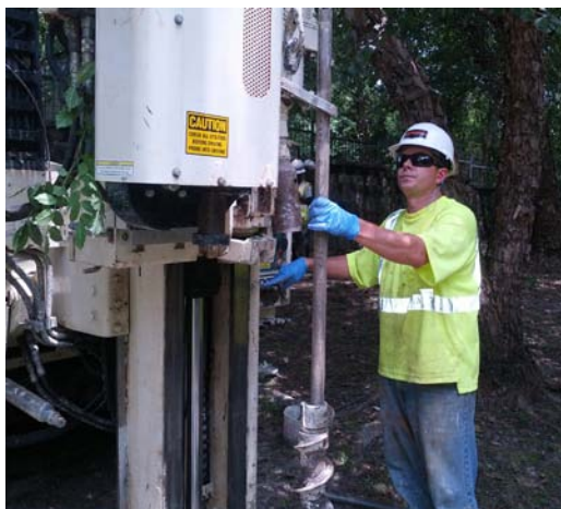
Dearal Rodgers, owner of Elite Techniques, Inc., retrieves an SPT sample via the augers on the Penn Branch project.
