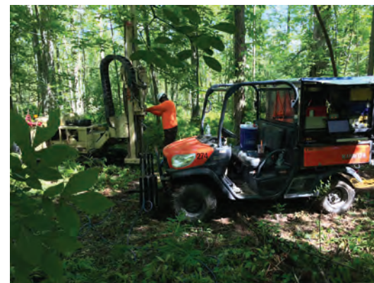
MiHpt Operator Jolaan Price is at the controls for Parratt-Wolff while taking their MiHpt tooling off road in Upstate New York.
