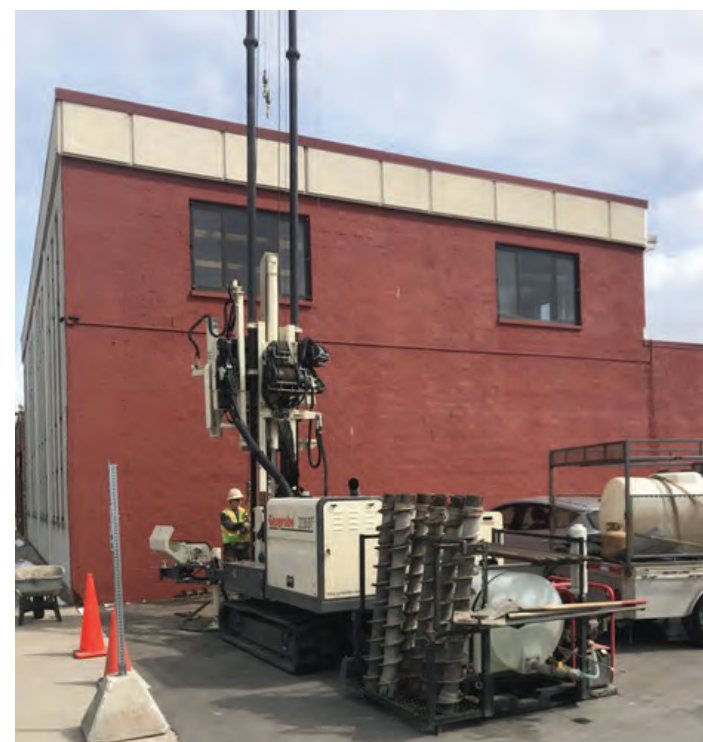
Shepler Well Drilling, Inc., completes split spoon sampling every 5 ft. in Traverse City, MI, as part of a geotechnical site investigation. Notice the customer built drop rack that utilizes the 3230DT rear blade to mobilize tools and supplies. The rack includes a power washer.
