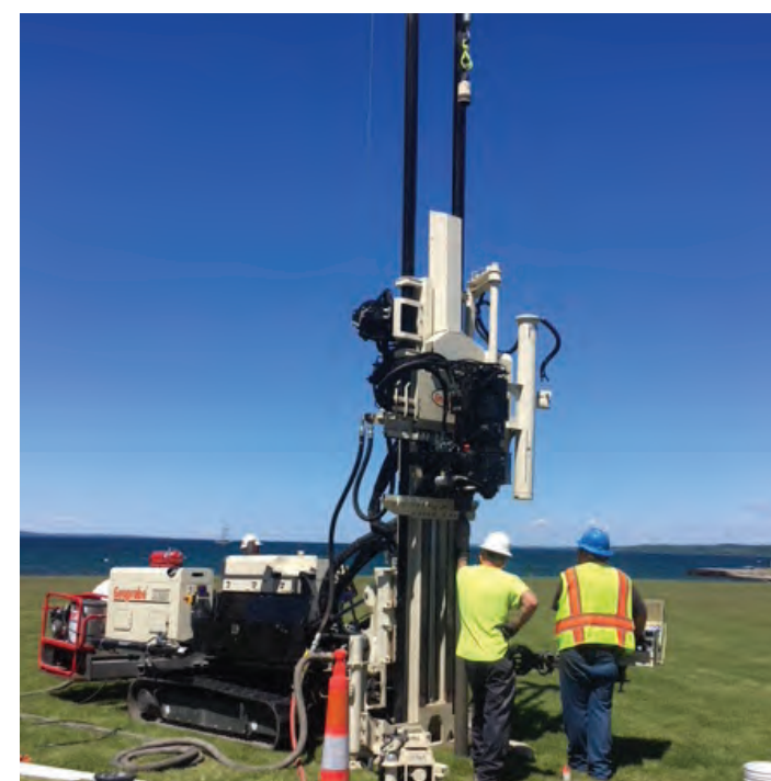
Shepler Well Drilling, Inc., President Randy Shepler and Operator Clint Bridson, advance 4.5 in. rods utilizing the GH70 percussion hammer to install wells.
