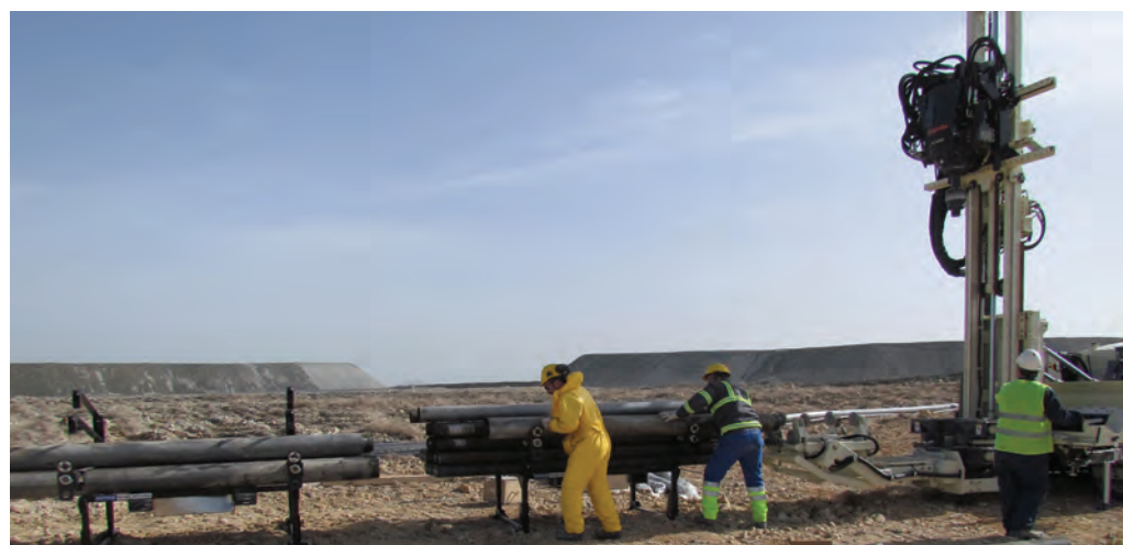
The Kisladag drill crew use two Geoprobe® Indexing Racks to position Geoprobe® 4.5 in. Heavy Duty (HD) sonic rods into the grippers of the rig-based rod handler on the 8150LS. Using the indexing racks and rod handler, the crew was able to trip 30 meters of 4.5 in. HD rods from the hole in less than 10 minutes.
