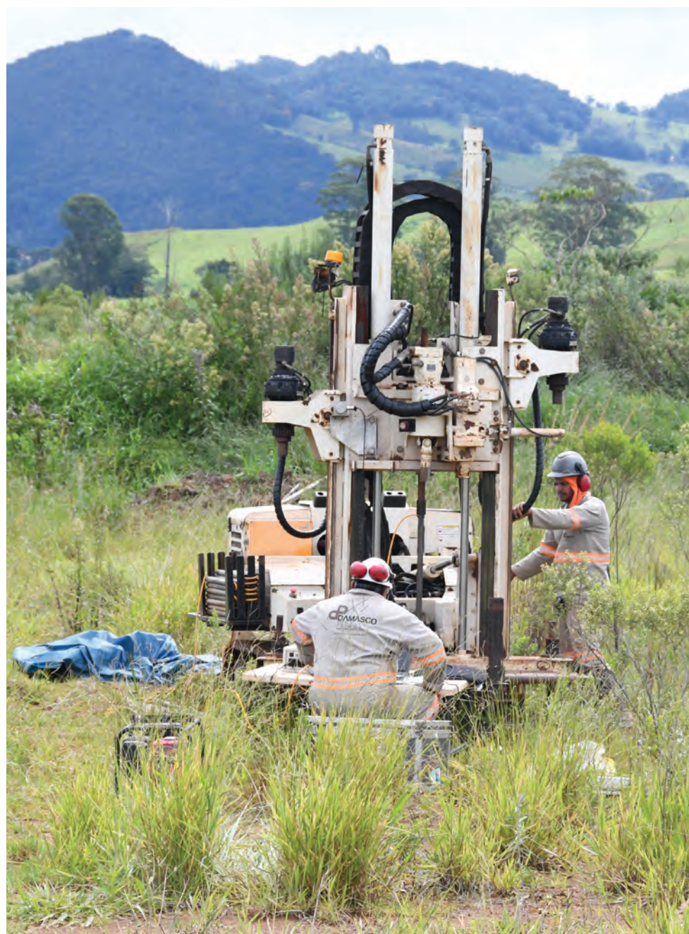
From left, Test Operator Jucelio Alencar and Drill Rig Operator Dorgival Sales perform a geotechnical site investigation near Poços de Caldas, a city known for its therapeutic hot springs and spas. Using their Geoprobe® 6625CPT and 7822DT machines, the Damasco Penna team sampled through soft clays up to 30 meters, collected rock samples, and performed everything from CPTU to mechanical SPT soundings.
