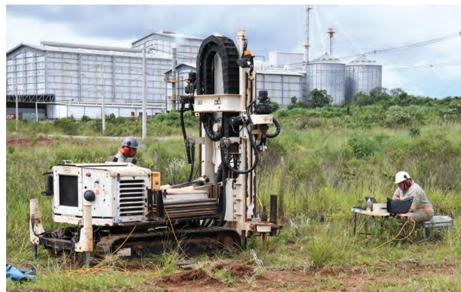
From left, Drill Rig Operator Dorgival Sales and Test Operator Jucelio Alencar perform CPTU tests using the Geoprobe® 6625CPT.
