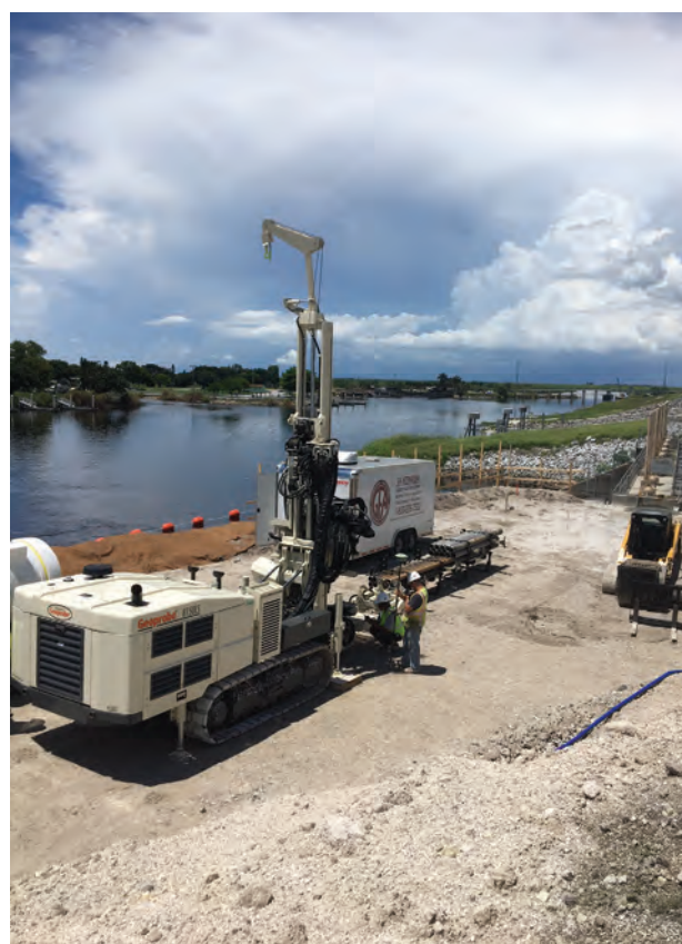
GFA International uses their 8150LS rotary sonic at the Herbert Hoover Dike, which is part of a rehabilitation project they’ve been working on since 2008.
