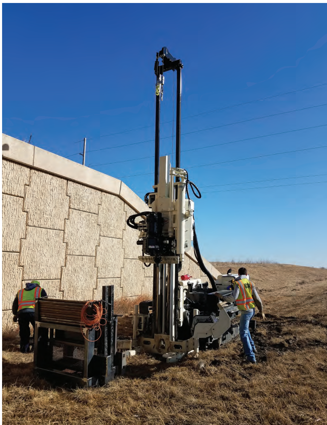
Top Right: (l to r) Driller Allen Hilgren and Engineer Alex Silvey perform CPT research for pile design at a bridge over Interstate 80 east of Lincoln, NE, using the 3230DT.
