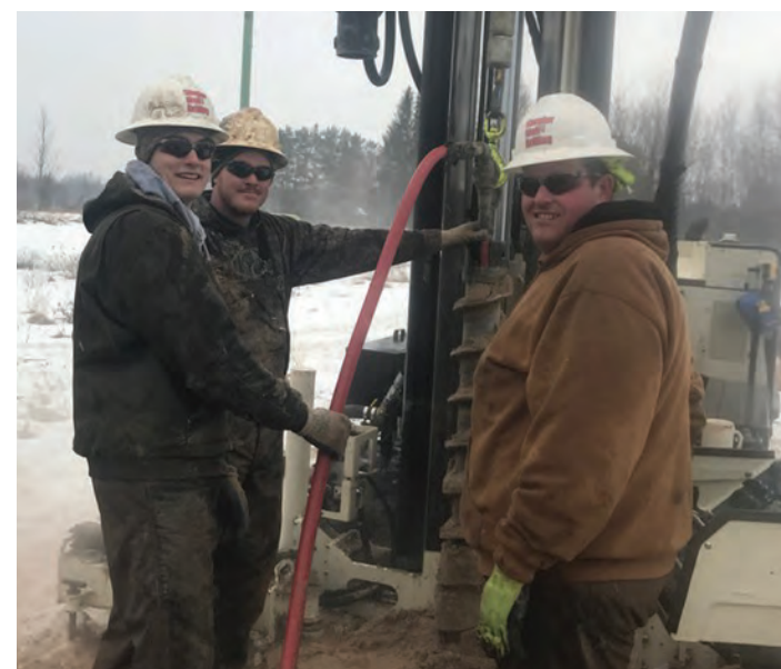
The Shepler Well Drilling crew, which includes Operators Cole Shepler, Darrin Mosher and Clint Bridson, use 4.25 in. hollow stem augers to 195 ft.
