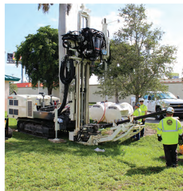
Driller John Holdsworth, Drill Helper Josh Perell, and Lead Driller Brian McCord set 2 in. wells to 220 ft. The 2 in. wells will be used for monitoring of salt water intrusion along the coast of Florida and aid the USGS and city managers in managing the water resources of the City of Hollywood, FL.
