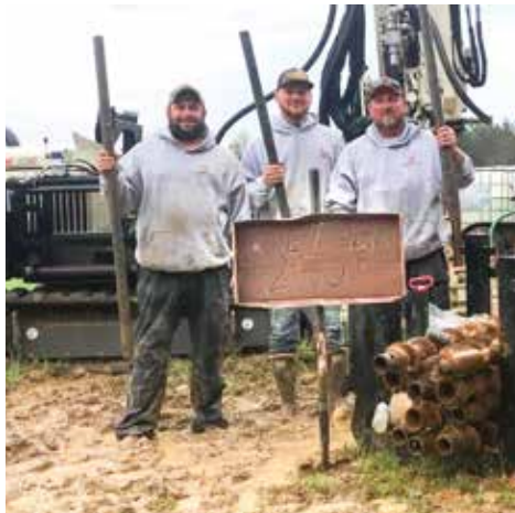
Above: David LeGrand, owner, and drill crew celebrate achieving a 250-foot rock core with the 3126GT. Below: Using their 3126GT, Catawba Valley Engineering and Testing successfully cored through granite/quartzite to depths of 200 to 250 feet.
