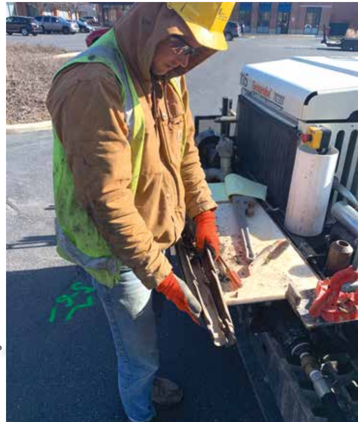
Top Right: Drill crews appreciate the reduced strain and self-adjusting capabilities when threading and unthreading rods when using the Geoprobe® spring assisted swivel lift cap. Bottom Right: Engineered features of the patented Geoprobe® interlocking split spoon improve field performance and longevity.
