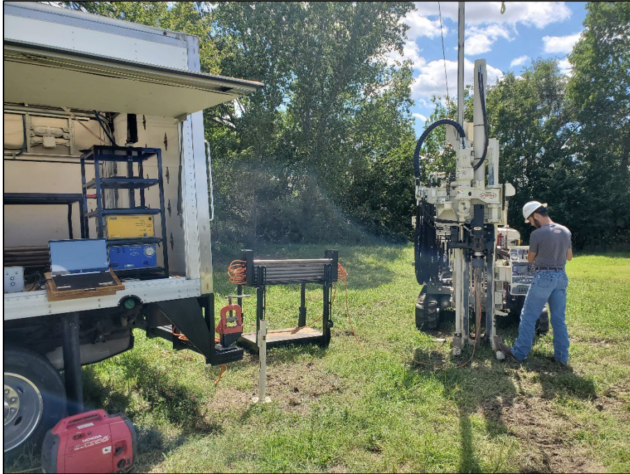
Figure 2: Operator setting up HPT Probe for advancement into the subsurface with a Geoprobe® 7822 machine. The HPT probe is advanced at 2cm/sec using the system hydraulics and probe hammer when required. Logs to a depth of approximately 60ft (20m) are usually completed in about one hour.
