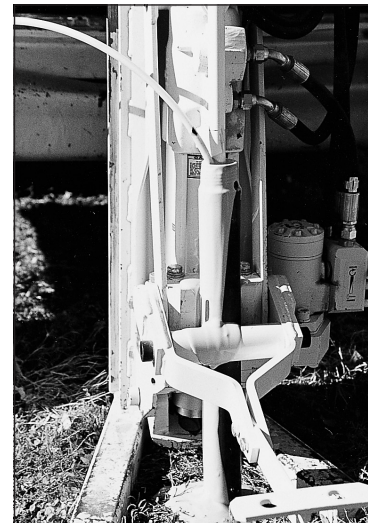
Figure 4.31. A grout machine and flexible tubing allow bottom-up grouting as the outer casing is retrieved.
