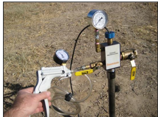
Figure 12: Setup for leak test and rising head tests with the pressure gauge and hand pump. The gauges are graduated in inches and centimeters of water pressure (outer and inner marks respectively). Close the inlet valve after pressurizing.
